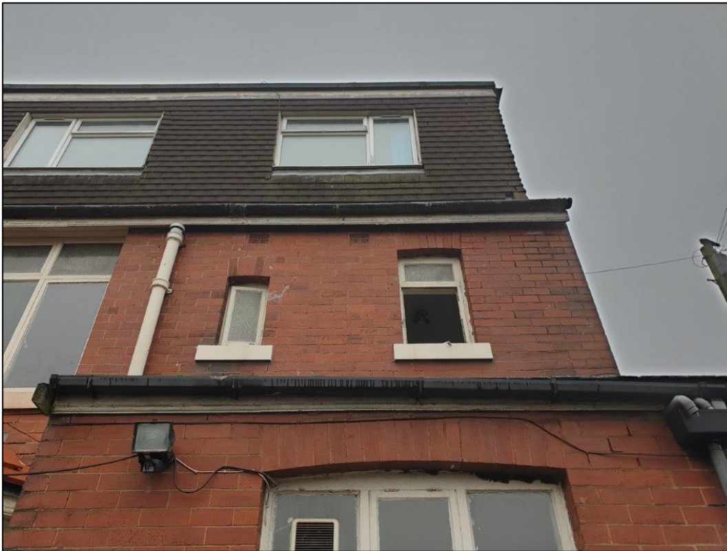
Image 5: First floor rear elevation with evidence of missing window
