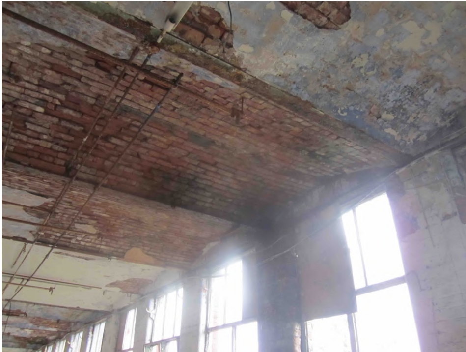
Photo 11 - Soffit to roof structure (photo at 3 rd floor level) by the southern elevation (water ingress appears to have eroded mortar)
