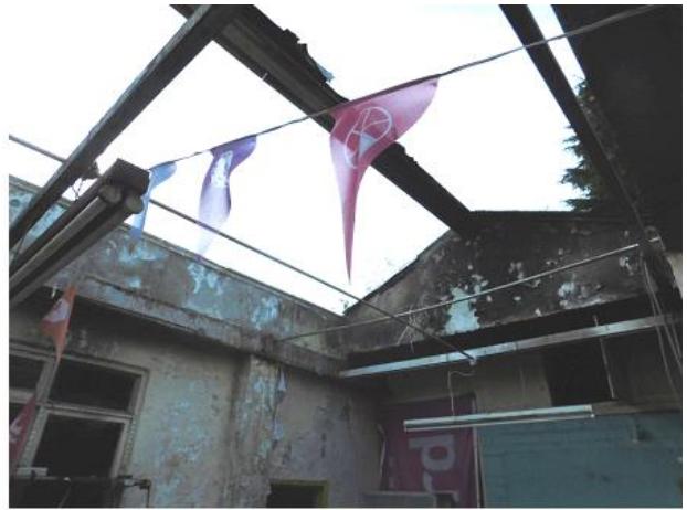
PHOTO 20 Missing Western Part of Building 2 Roof
