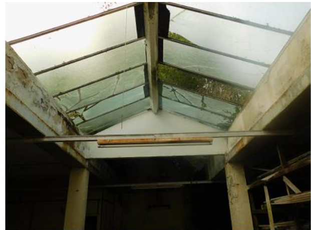
PHOTO 26 Missing Central Building 2 Roof
