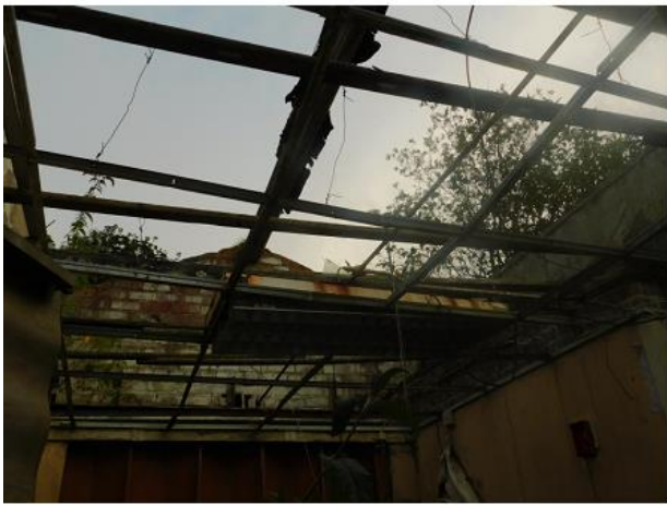
PHOTO 21 Missing Central Part of Building 2 Roof
