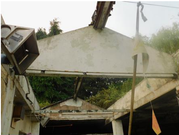
PHOTO 25 Missing Western Part of Building 2 Roof
