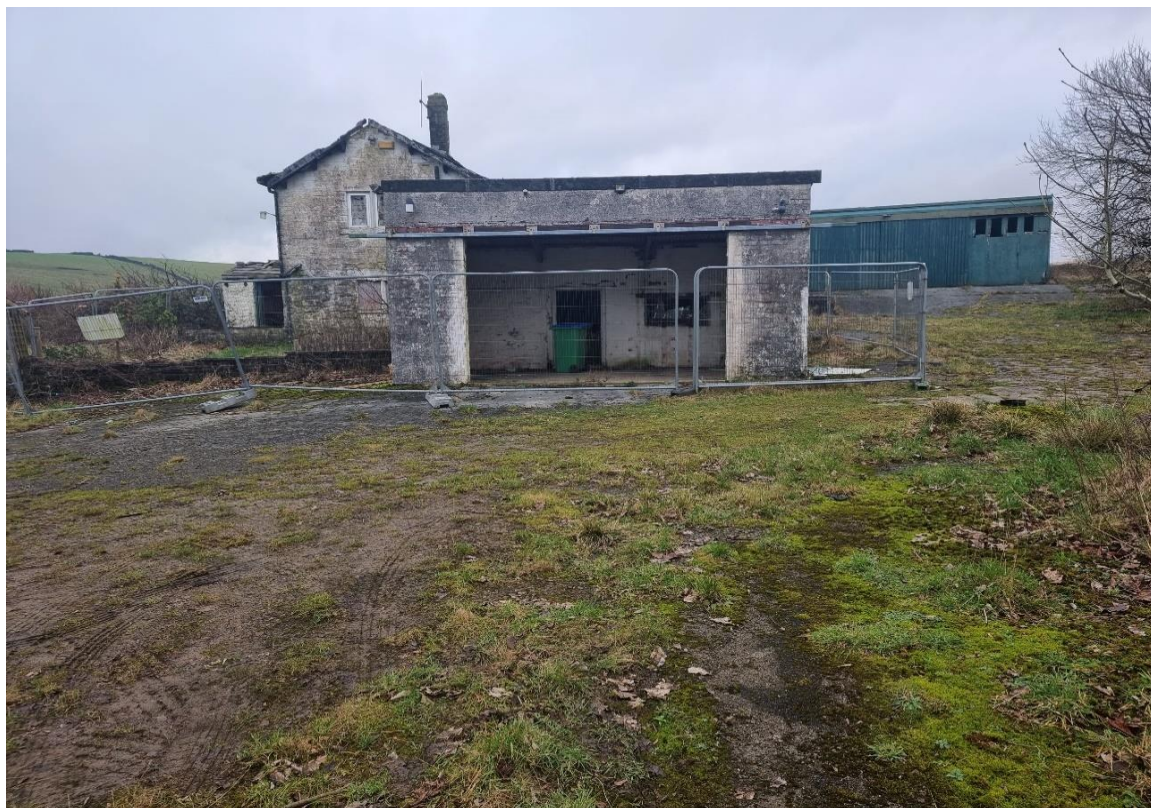
Derelict Longley Hey Farmhouse side view with tarmac surface in foreground.
