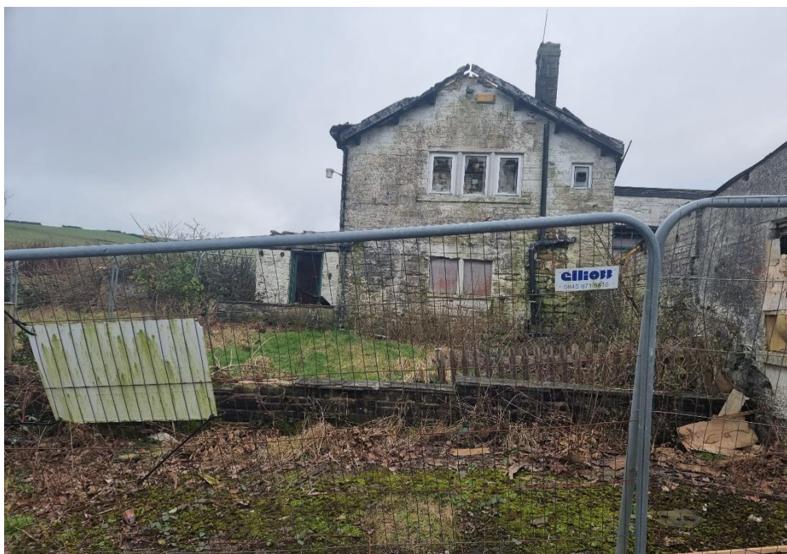
Derelict Longley Hey Farmhouse side view with Heras fencing in foreground.
