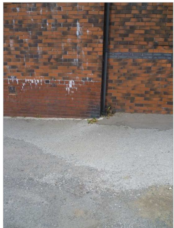
Neighbouring property free discharge onto access lane
