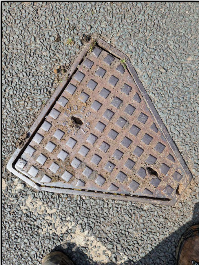
S2 Seized Manhole Cover
