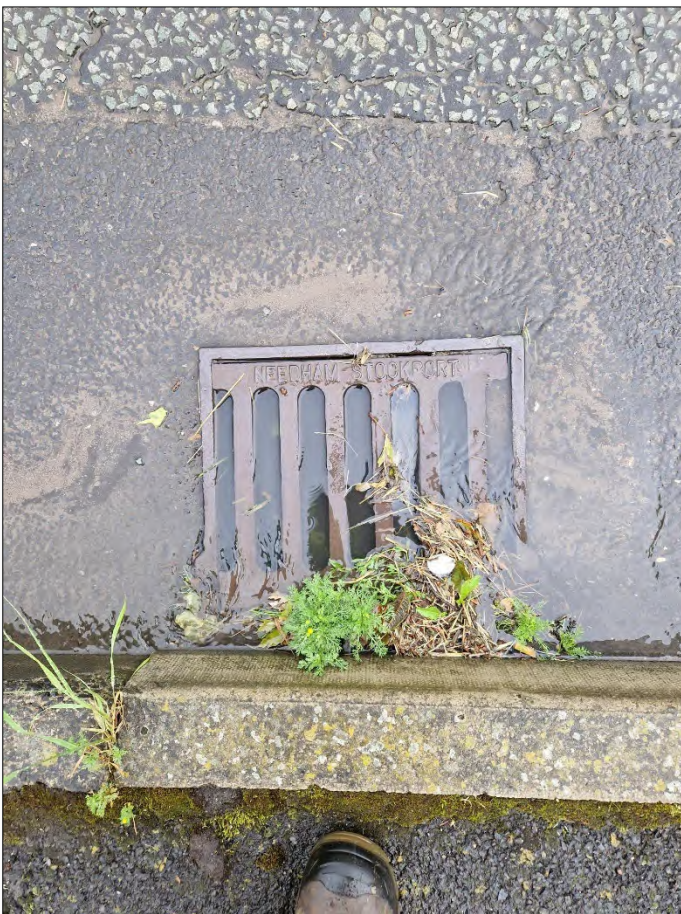
Road Gully Condition Example
