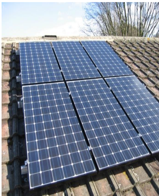
Figure 5 - Photovoltaic array on a pitched roof
