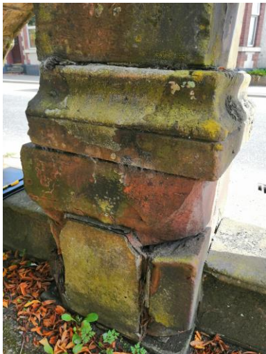
Stone number 6 - Plinth dislodged. Moulded profile. No work required.
