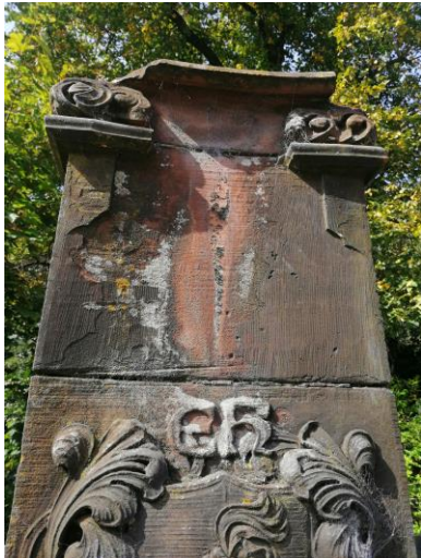
Stone number 2- Radius profile to front face, corner mouldings. No work required.
