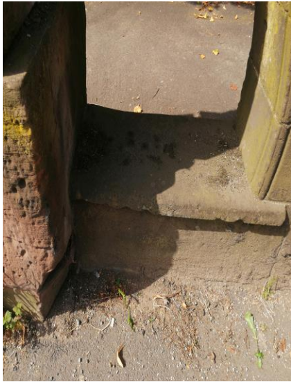
Stone numbered 38- Plinth stone profiles missing on 2 faces. No work required
