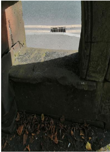
Stone number23- Plinth stone profiles missing on 2 faces. No work required.
