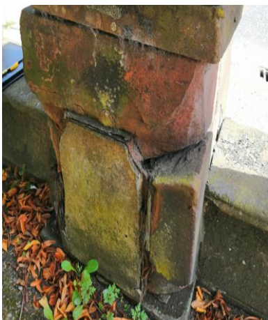
Stone number 7 - Radius profile to front face. Multiple fractures to rear face and sides. Replace stone like for like 600x 600 x 640.
