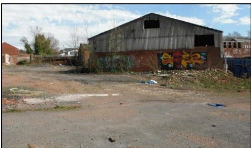
Asbestos sheeting to numerous buildings across Site (Building 4).
