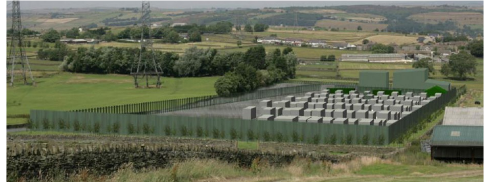
Harrop Lane BESS, Bradford (Greenbelt) - 24 Power Limited
