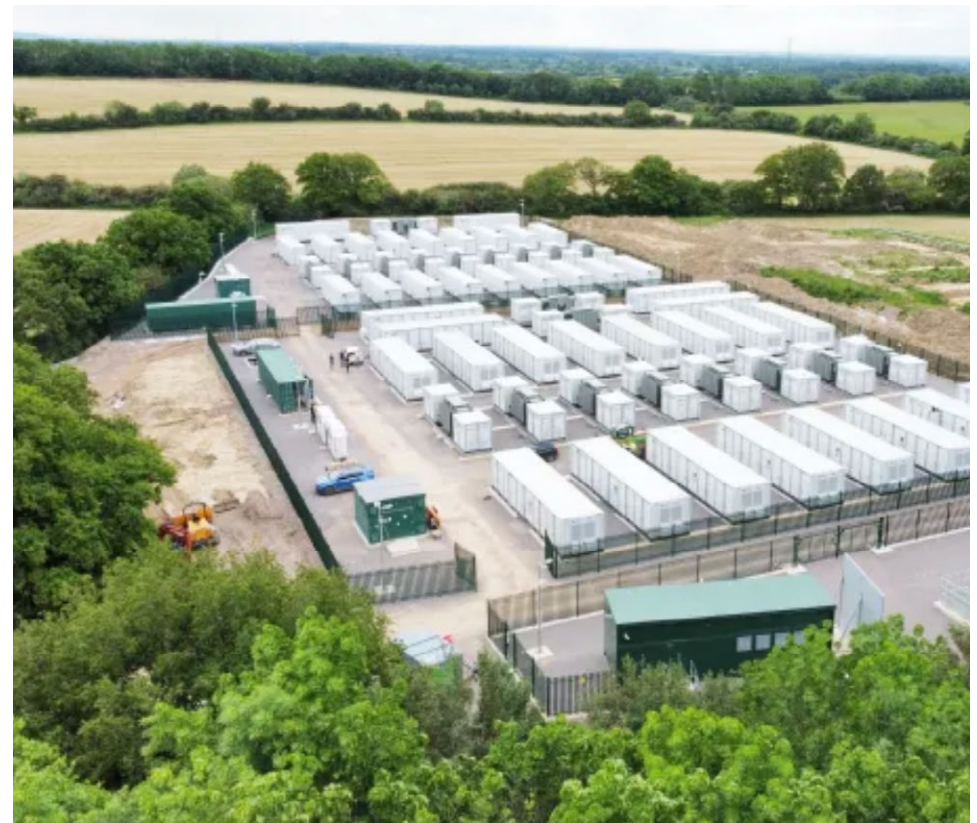
Minety BESS, Wiltshire - Penso Power
