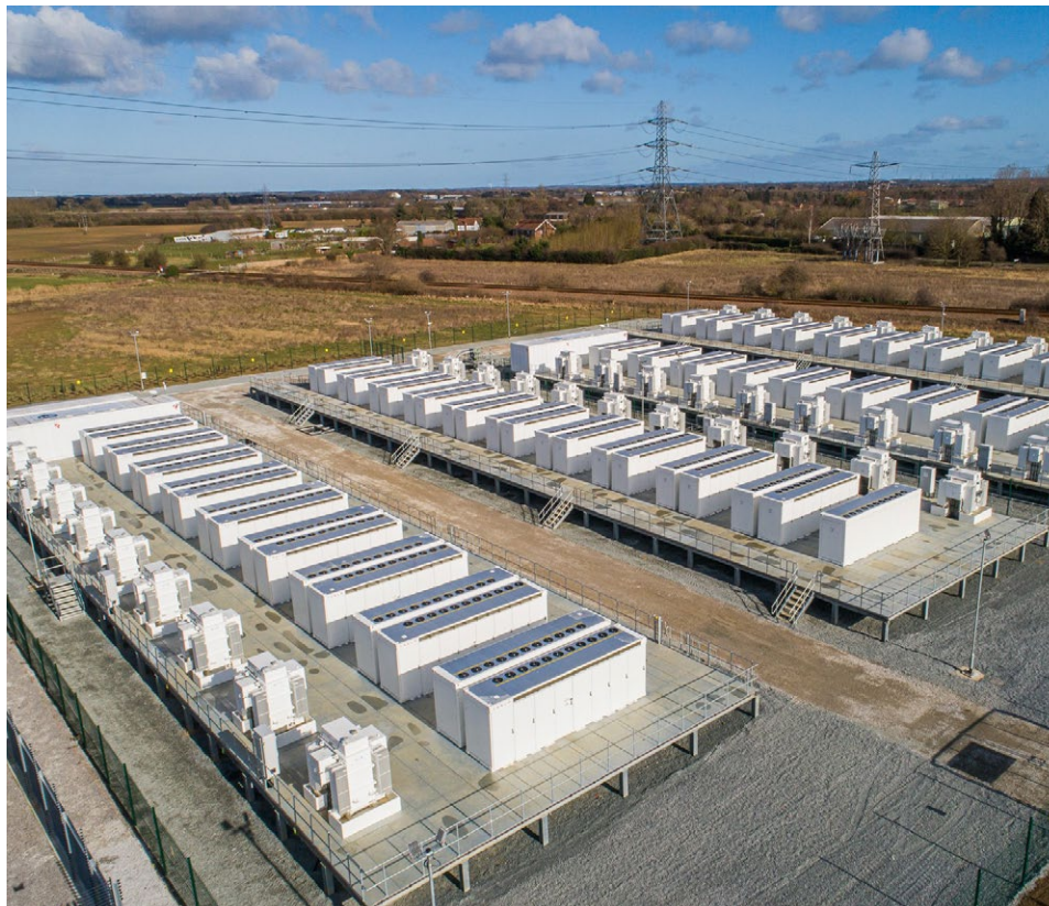
BESS, Pillswood - Harmony Energy
