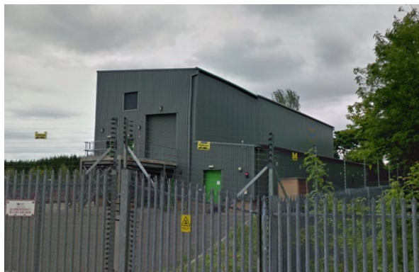
Equipment enclosure - Rochdale Power Station - metal cladding
