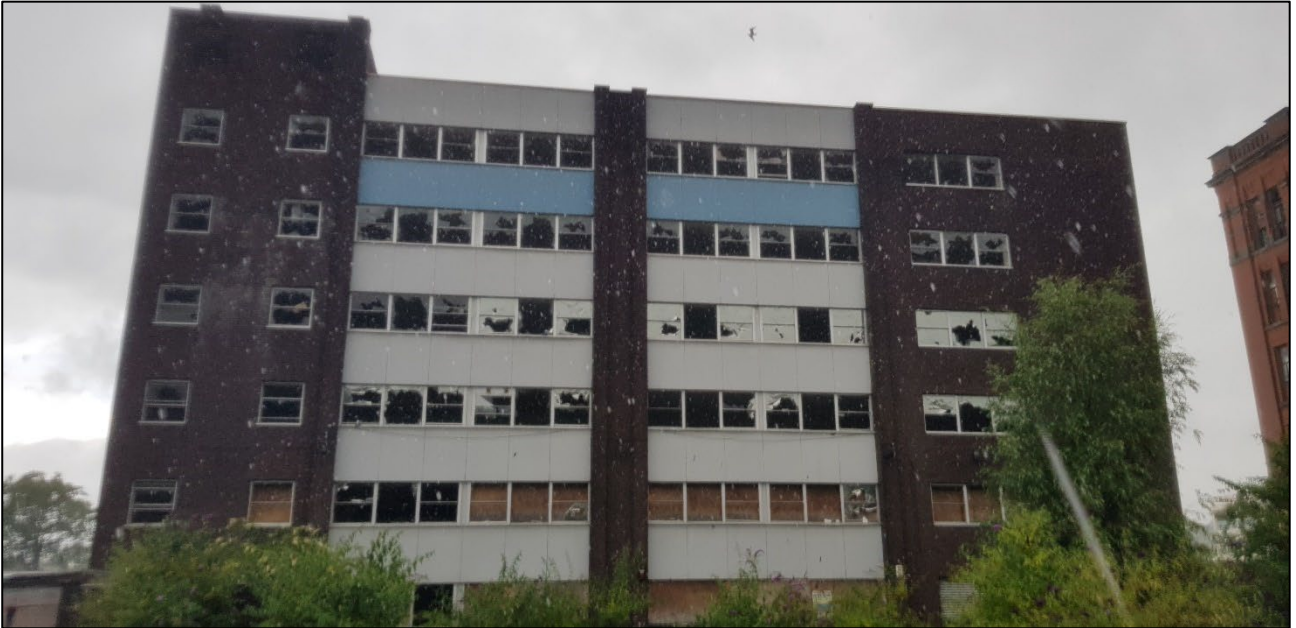
Photo 03. Abandoned apartment (u1b5)
