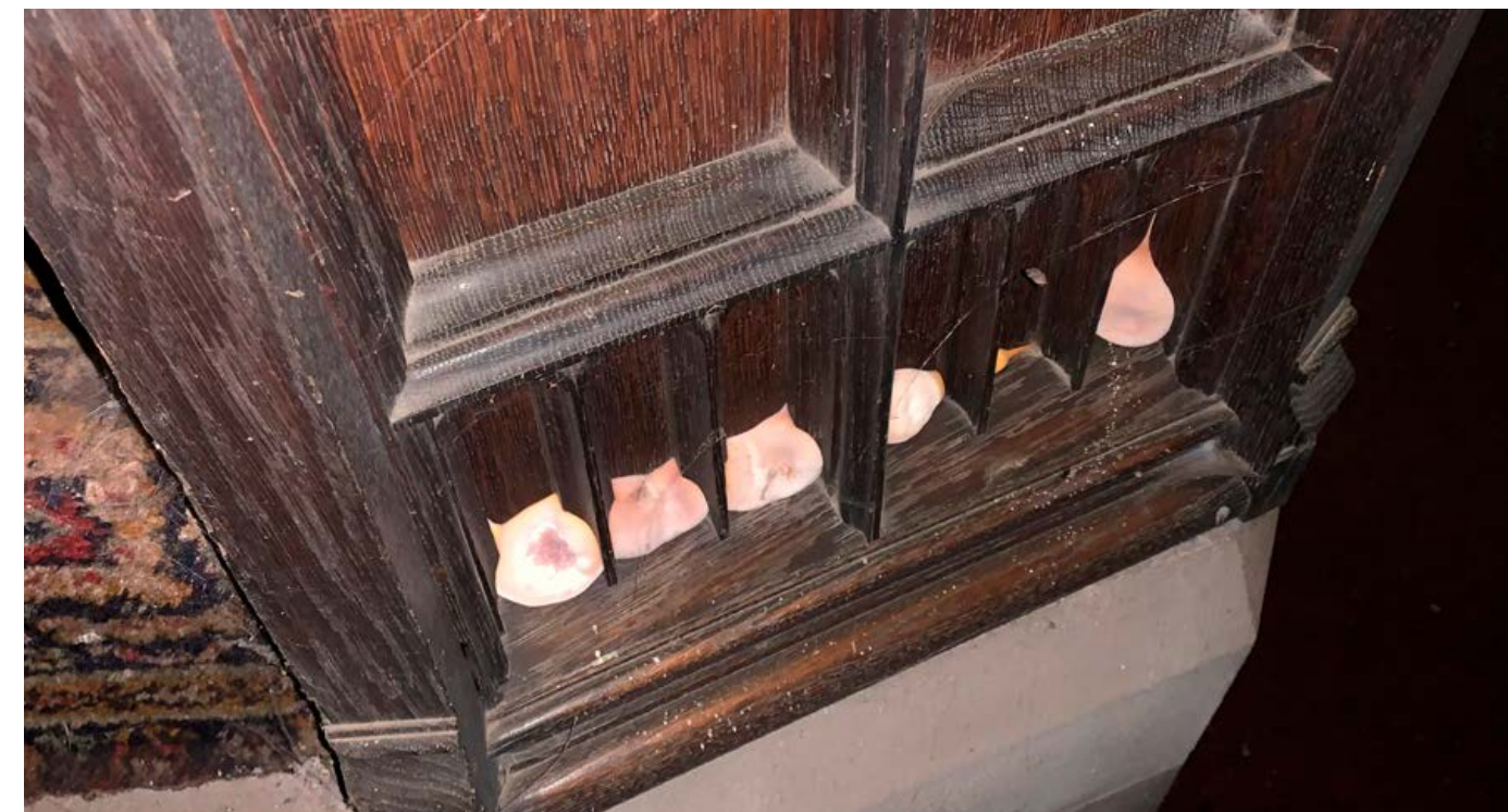
Figure 27 Images of Dry Rot Fungus on Pulpit
