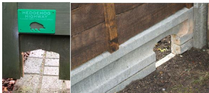
Insert 6: Showing wildlife access gap within fencing
