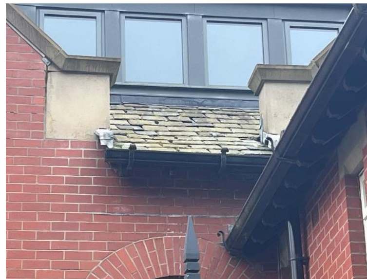
Photo 2: B1 – gaps between roof tiles – northern elevation.
