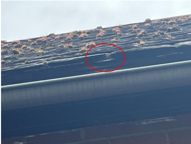
Photo 7: B2 – gap between tile along western elevation.
