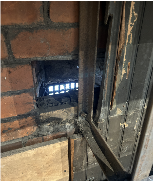
Image 02/04 - Closer look at vent position, brickwork opening and grille height. Grille sits directly behind existing brickwork meaning (cold) air needs to rise in order to enter space. S/o in brickwork for air movement is located at a higher level to external grille.
