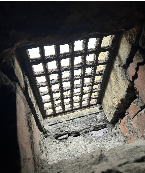
Image 03/04 - Photograph from within cavity looking at ventilation grille.
