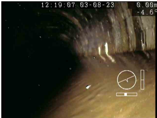
MH3X_1979f13f-2cef-4281-873c-6da0f7b91a3c_20230807_1 44220_784.jpg, 00:00:30, 0.50 m Settled deposits, fine, 25% cross-sectional area loss
