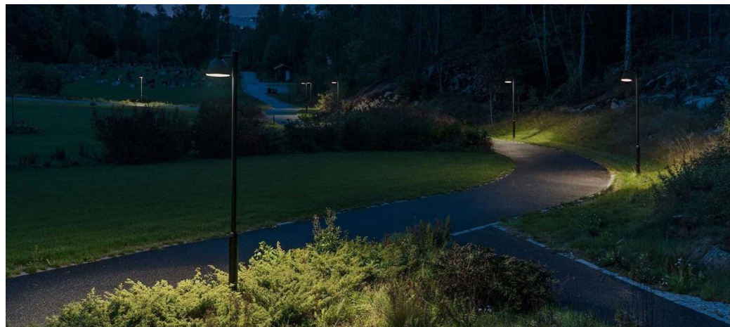
Column mounted lanterns illuminate pathways
