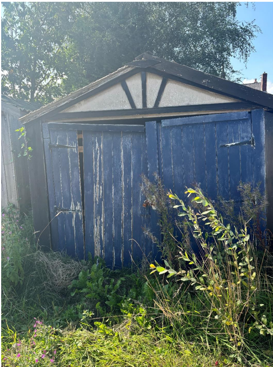
^ Figure 5.1: Photo of one of the dilapidated and unused garages on Church Avenue Plot.
