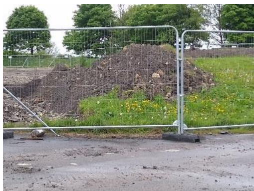
Photograph 3: Materials not stored appropriately.
