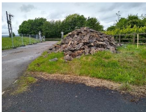
Photograph 2: Materials not stored appropriately.
