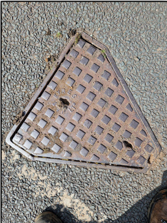
S2 Seized Manhole Cover
