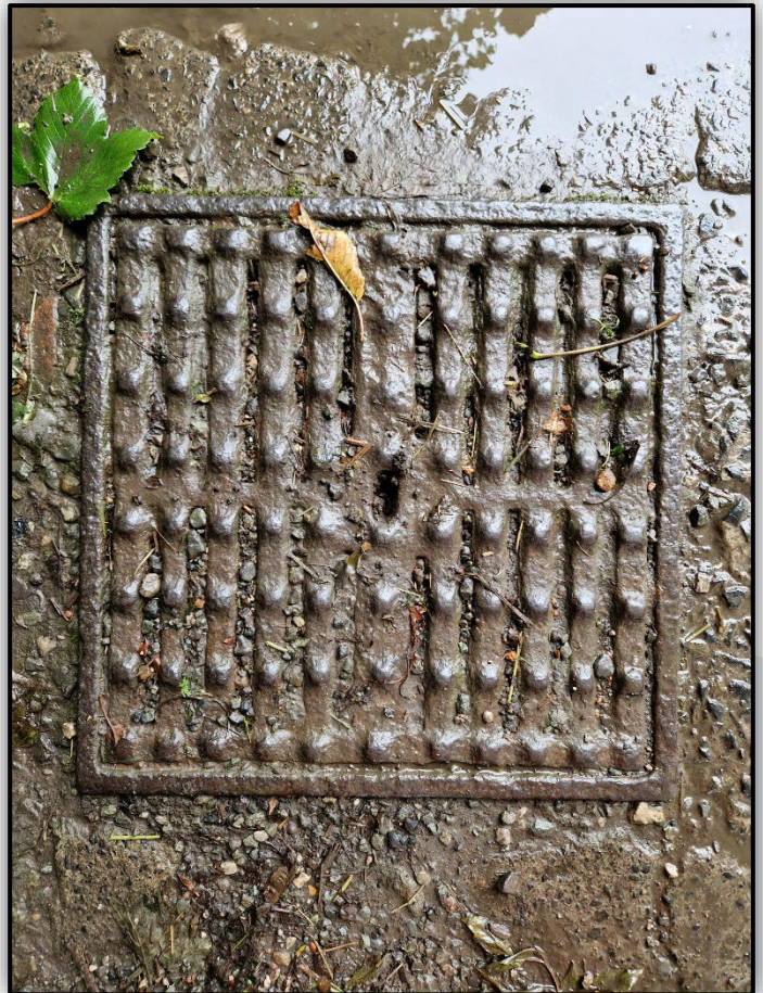
C5 Seized Grated Manhole Cover
