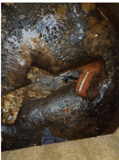
FWMH5 RAGS CAUSING BLOCKAGE
