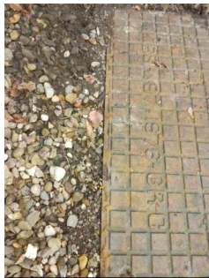
FWMH1 DEFECT SEIZED
