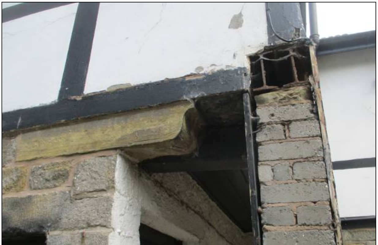
15. Corbel supporting the jetty stops short and appears to have been inserted
