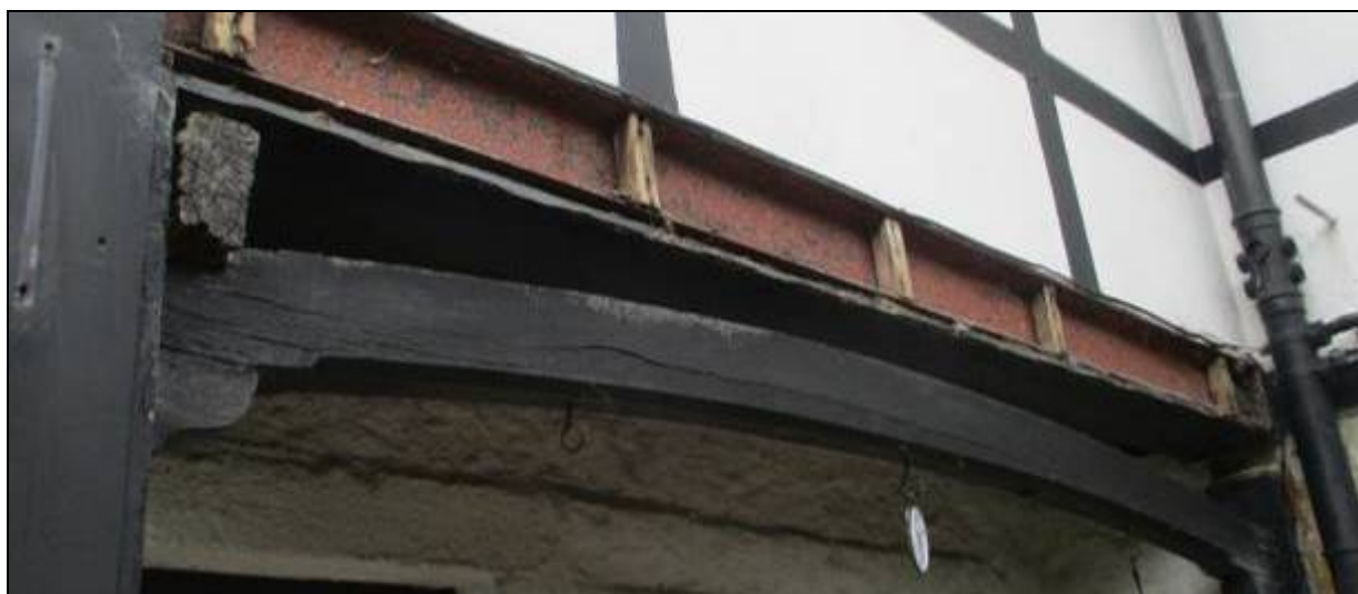
16. The arched beam beneath the jetty serves no structural function
