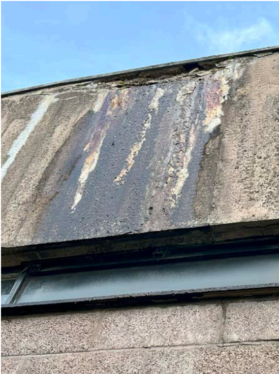
23 View of Damaged Concrete Ring Beam
