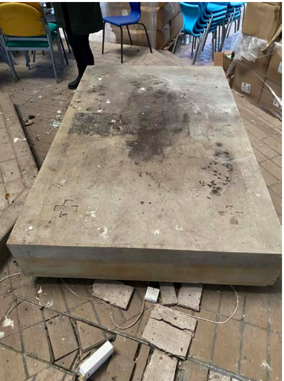
125 View of displaced Sanctuary Altar stone
