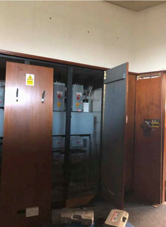
148 Electrical Cupboards in Sacristy
