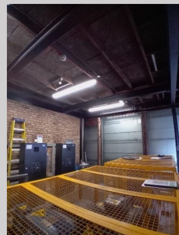
Photograph 19: Wiring room, block B
