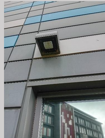
Photograph 17: Lighting block A
