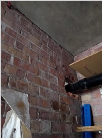
Photograph 26: Gaps were present in the internal walls between the garages.
