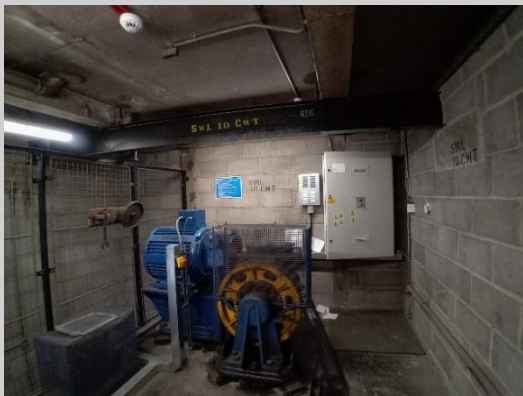
Photograph 18: Winch lift room on the roof of Block A.
