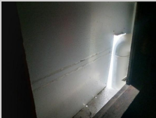
Photograph 22: Water tank room, block B. Potential access for bats.
