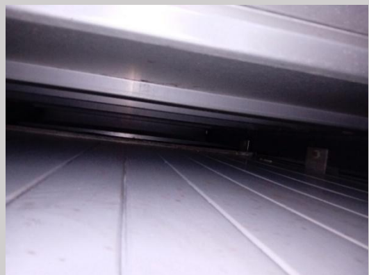
Photograph 23: Water tank room, block B. Potential access for bats.
