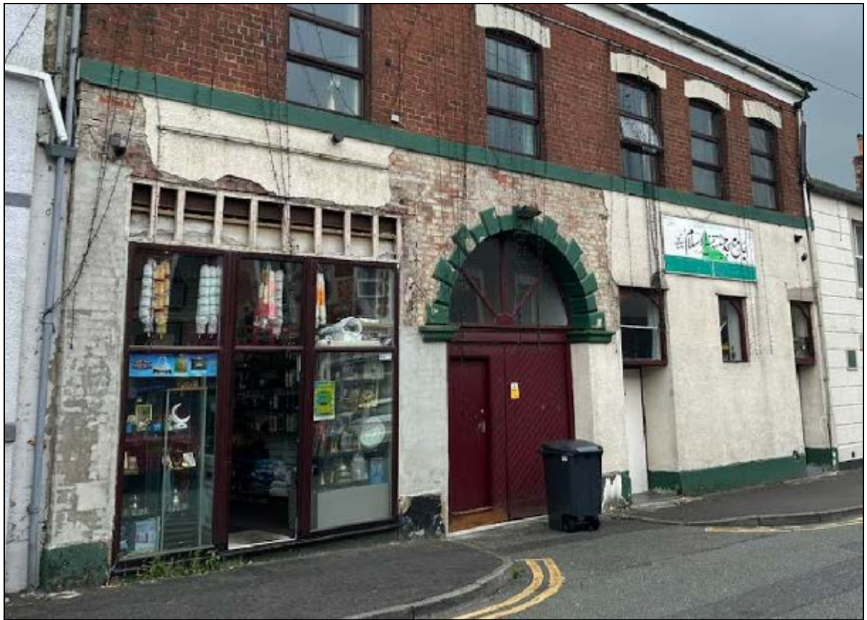
4. The property has been altered over time, with ground floor render and a new shop front
