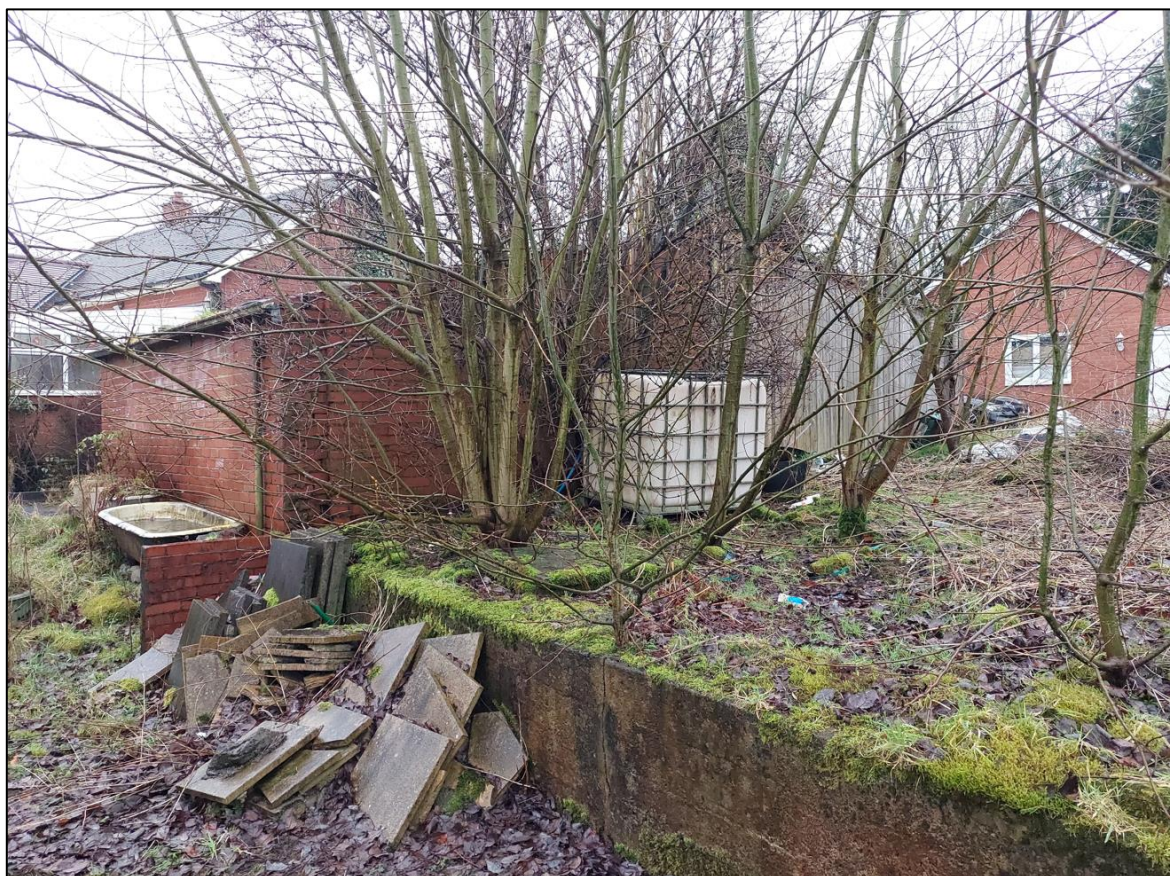
View of Dilapidated Outbuilding with Dwelling and Garage in Background (Facing South East)
