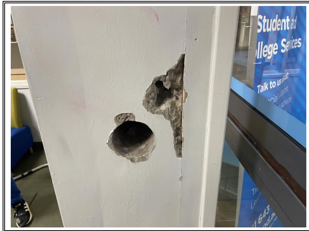
Core 1 – Location D – Column, west face Offset 170mm from north edge; 1280mm from ground level
