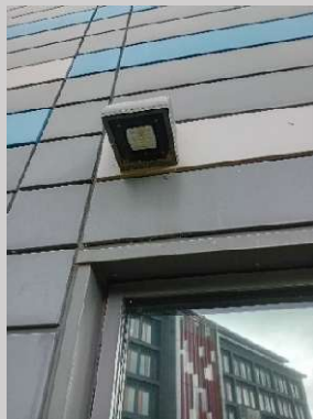
Photograph 3: Lighting on ground floor of Block A.
