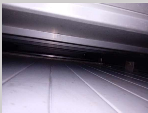
Photograph 10: Water tank room, Block B. Potential access for bats.
