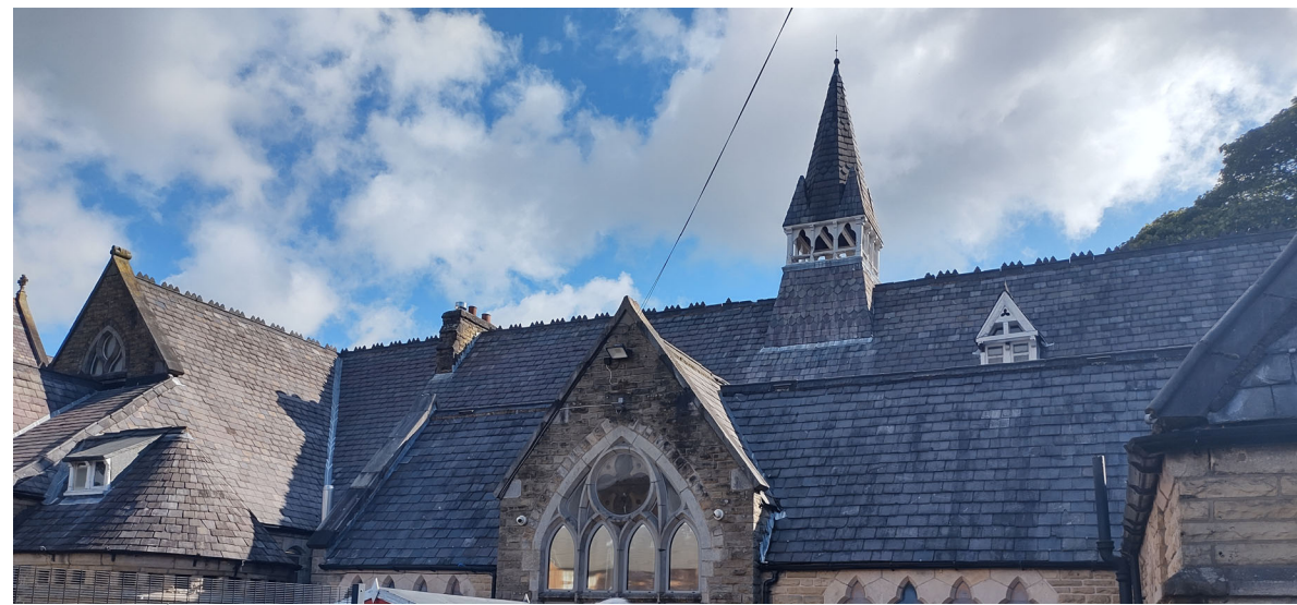
Broken Ridge Tiles mainly around Cupola
