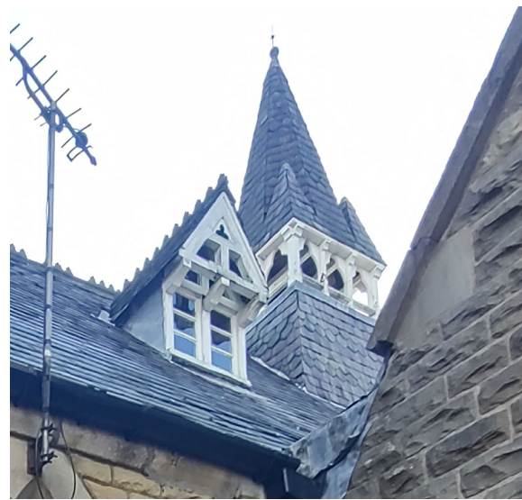
C3 Dormer window woodwork requires repainting
