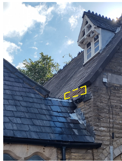
Additional guttering required in this area
