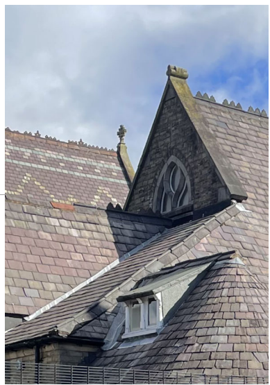
Significant Ridge tile damage in this area
