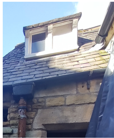
G1 Non-Gabled 'Shed' Dormer Windows require re-felting
