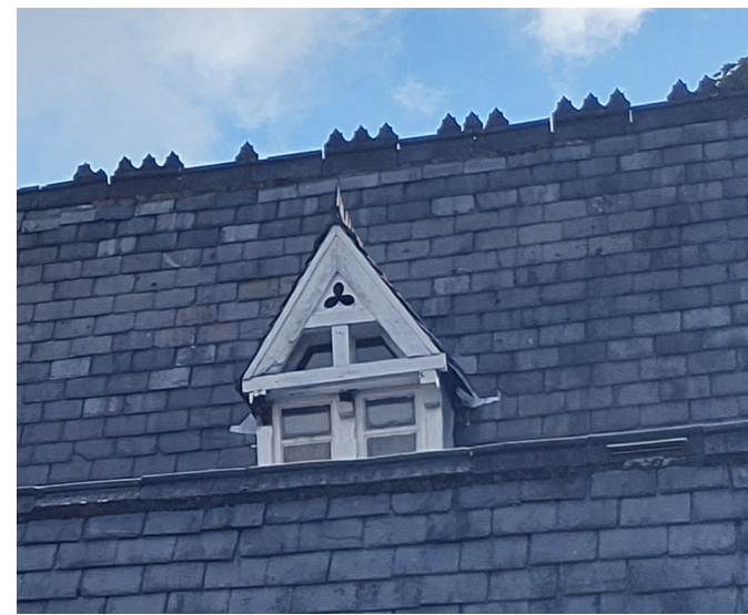
C4 Dormer window woodwork requires repainting
