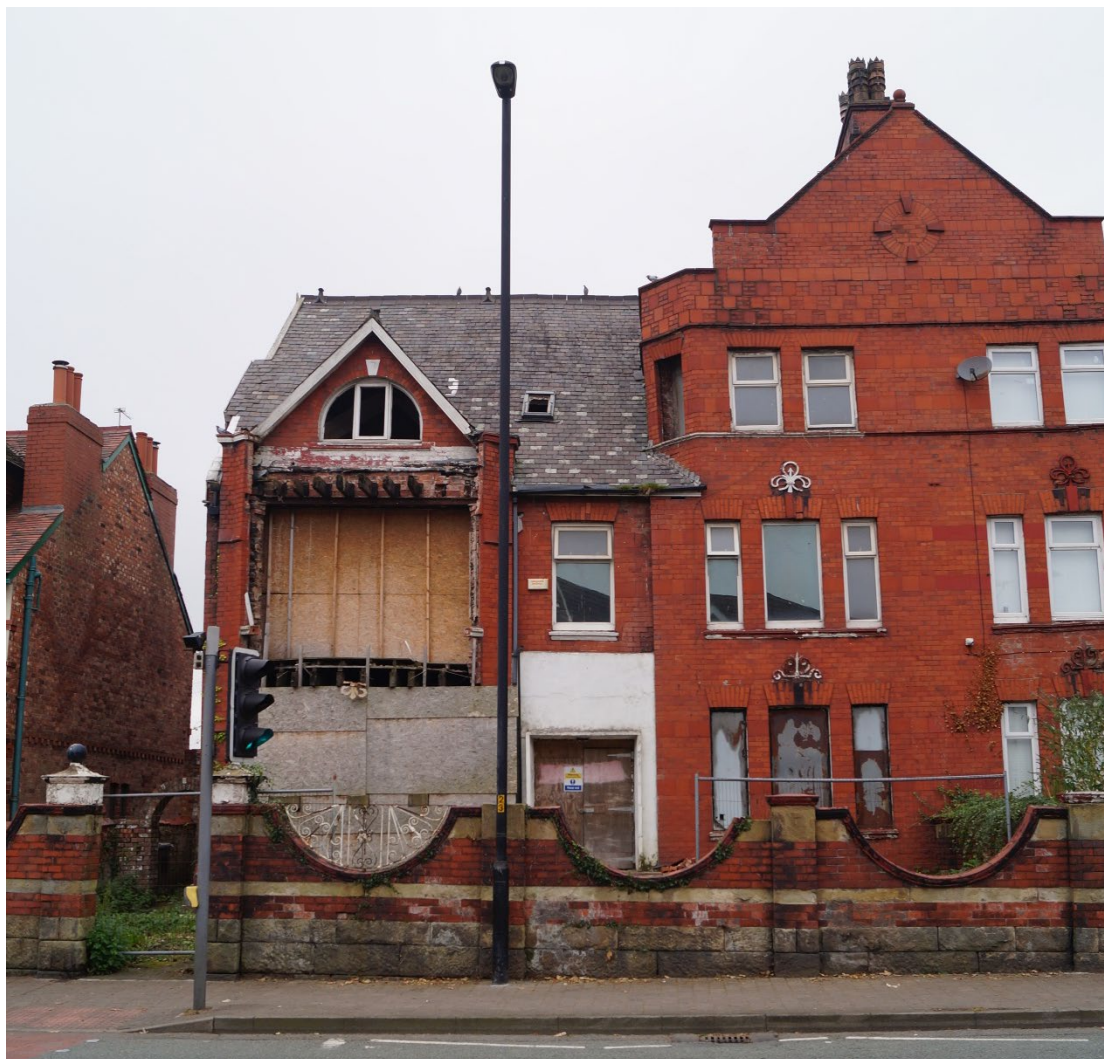
Fig.32: Front elevation showing the condition of the building with front bay removed and security boarding to doors and windows. This view shows the boundary wall to the street.
