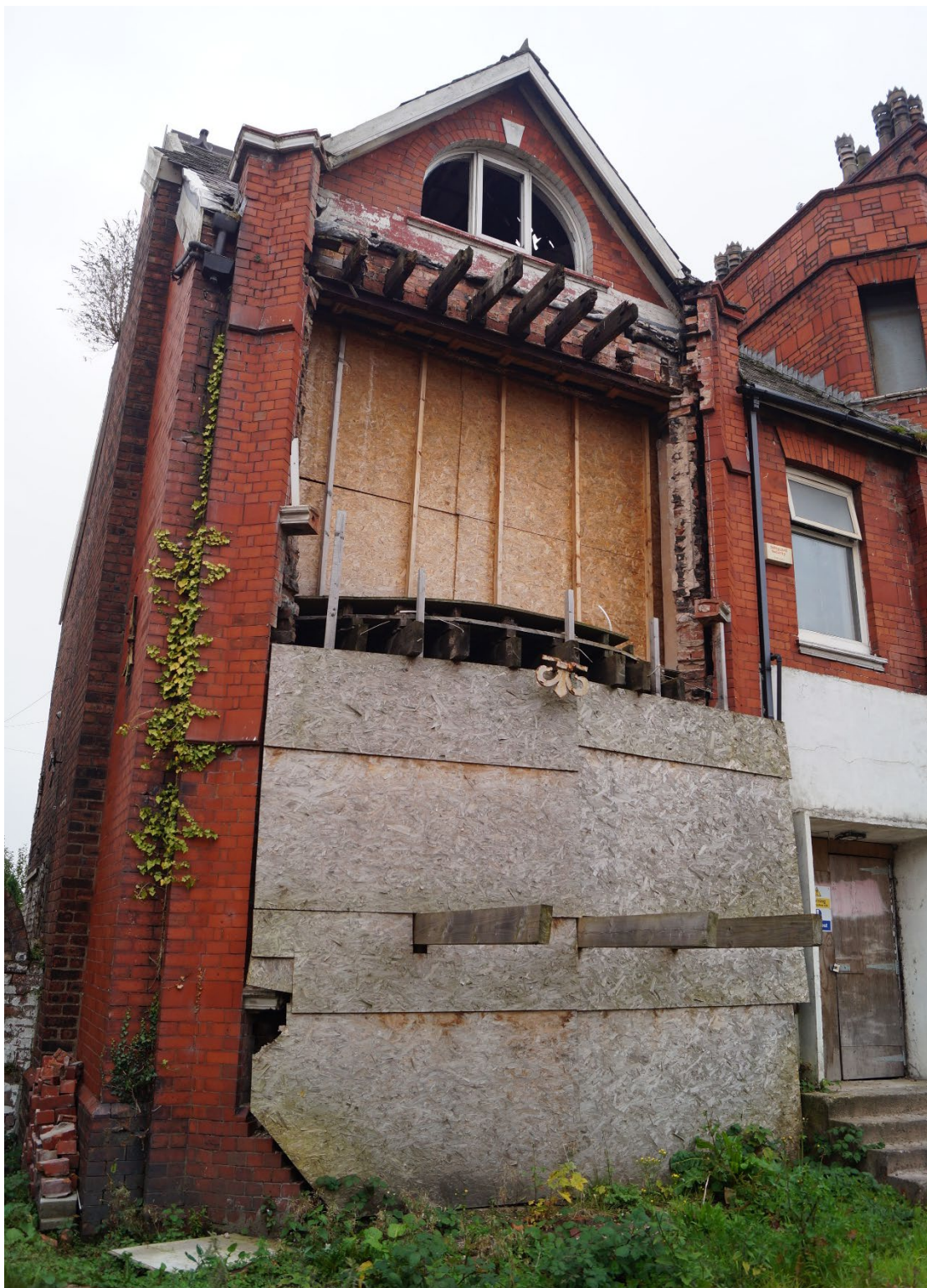
Fig.4: View of the front elevation showing the hoarding to the location of the dismantled two storey bay. The projecting timbers to the former flat roof in front of the arched Diocletian window are a concern, as are the exposed joist ends to the first floor. High level vegetation to the side elevation was identified as urgent work to prevent further deterioration and the potential for masonry falling from the building.
