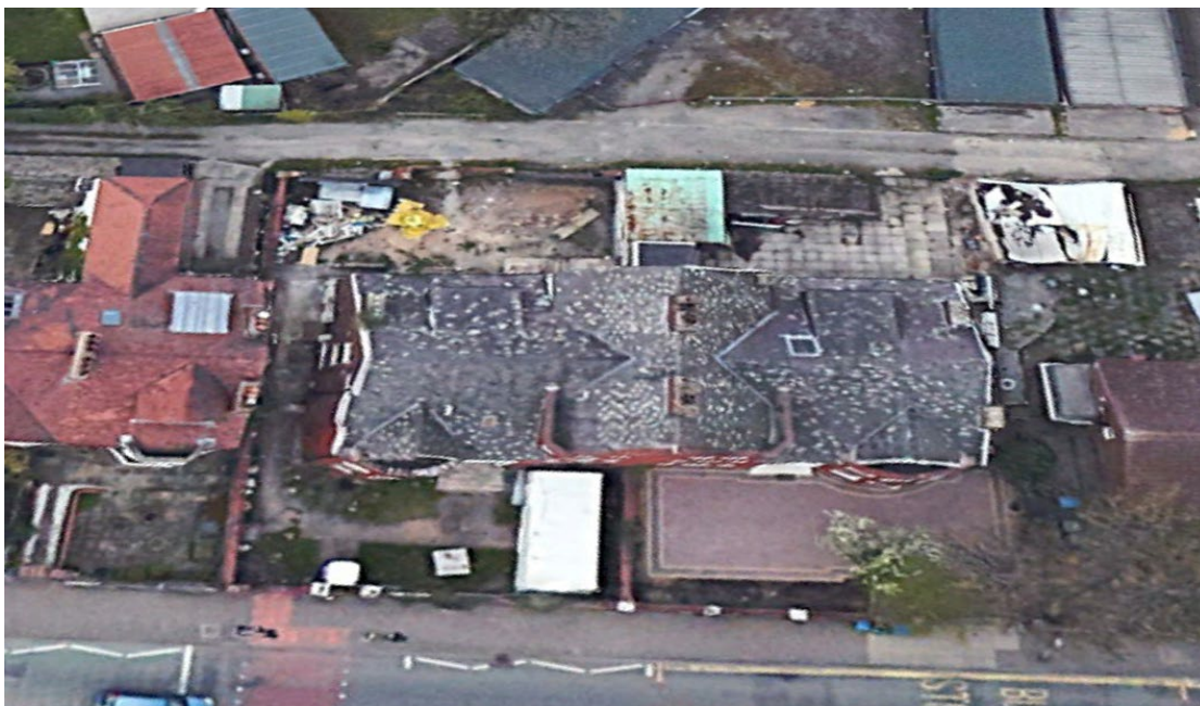
Fig.25: Satellite image from March 2021, the bow window is still visible in this image. Roof repairs appear to have reduced the freckled appearance of the polychromatic slate roofing, which appears as a more even grey colour to the section behind the bow window gable.
