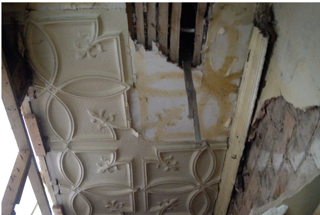
Fig. 11: Internal view of decorative ceiling to ground floor stair well to be retained and carefully repaired in situ.
