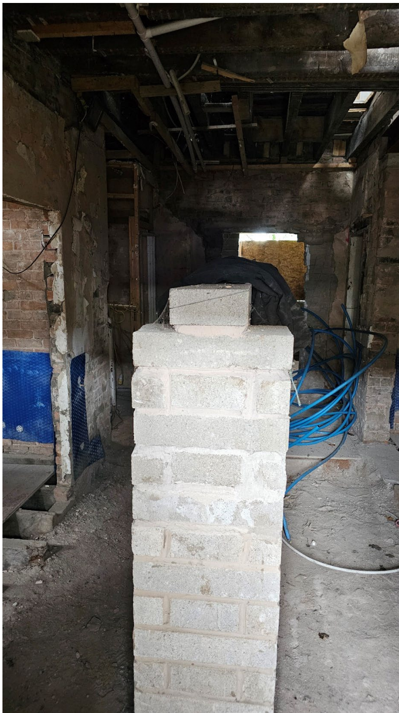
Fig. 10: Internal view of the partially constructed party wall to the entrance hall at ground floor level. The concrete blocks have been laid flat instead of in the normal vertical orientation.
