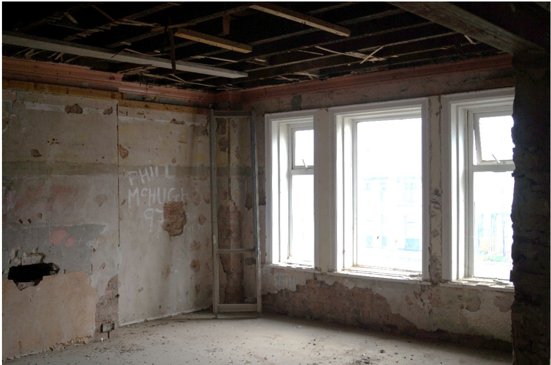
Fig.7: Internal view of the first floor to the front showing the bare walls and removed ceiling. The opening in the wall on the lefthand side is a former fireplace position.
