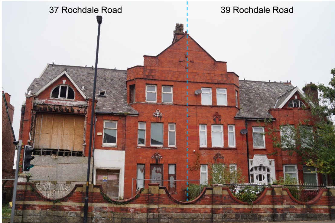
Fig.2: Site photograph with no.37 Rochdale Road on the left and no.39 on the right, with their shared gable in the centre. The party wall is indicated by the dashed blue line. The poor condition of the building is evident with the dismantled bay and boarded up doorway.
