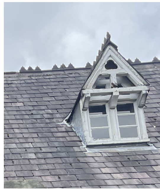
C1 Dormer wooden damaged; will require replacement sections
