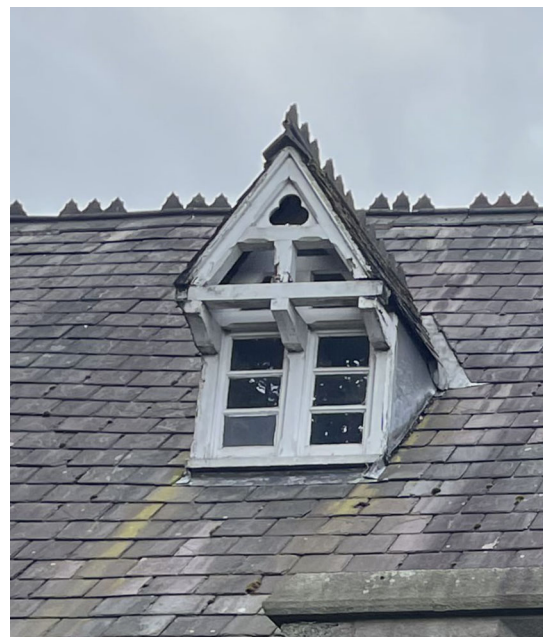
C2 Dormer wooden damaged; requires further inspection
