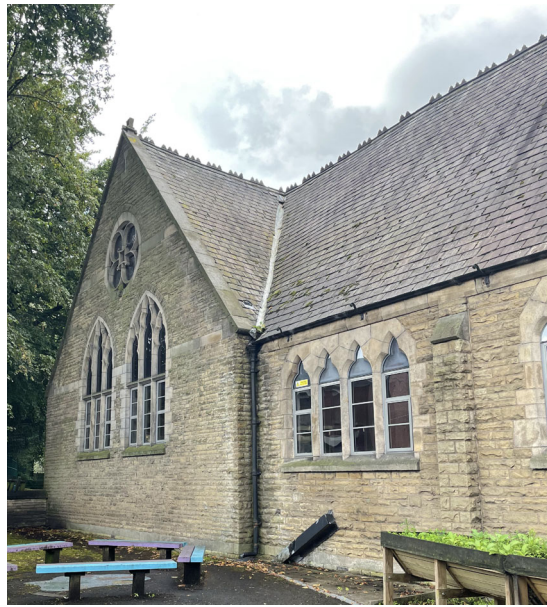
Multiple damaged Ridge Tiles
