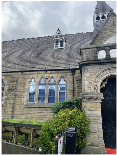
Ridge Tiles damaged near Cupola
