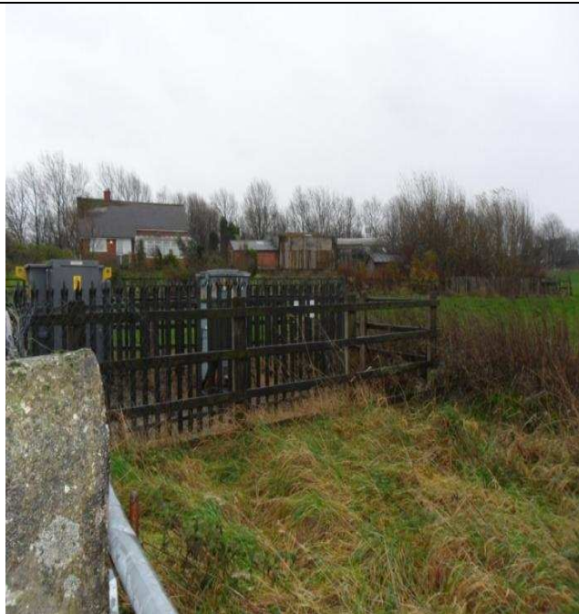
Photo 1: Electrical sub-station located along eastern site boundary.
