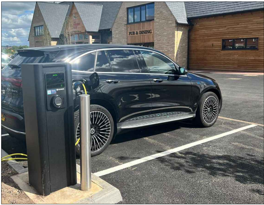
EXAMPLE OF DUAL PILLAR CHARGER
