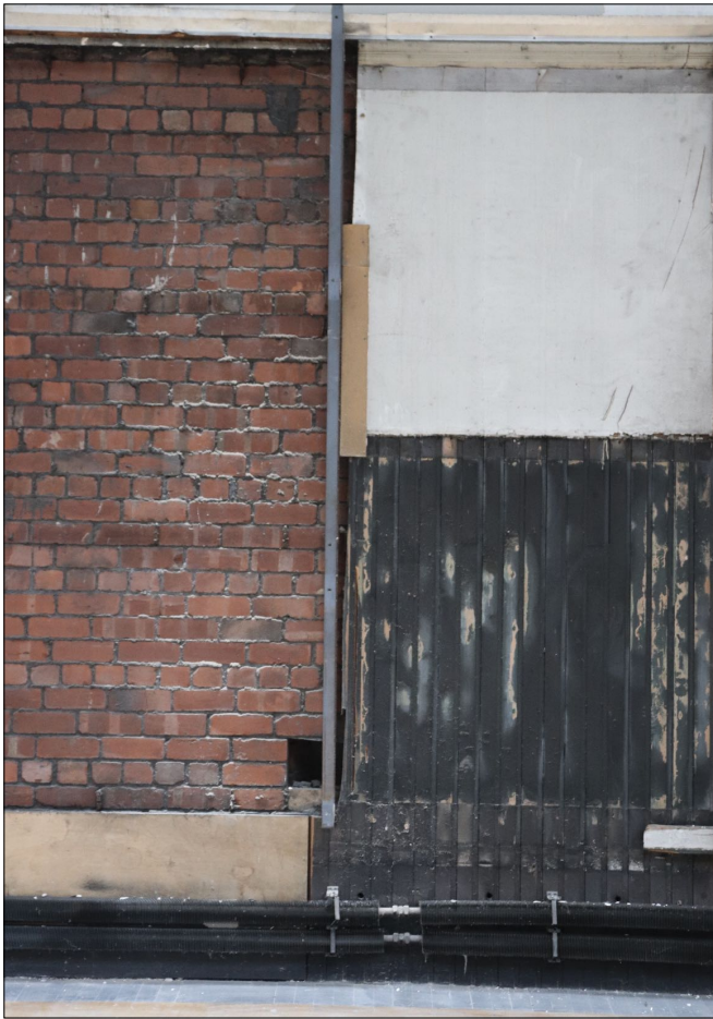
Image 02/04 - Example area where existing wall coverings came loose following exhibition board removal due to deteriorated fixing points / general poor condition. Brickwork and (one of many) existing ventilation point became exposed.
