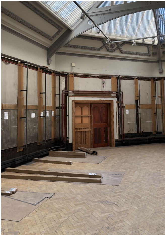
Image 04/04 - Image highlighting numerous locations where T&G has been cut to allow for metal frame fixing into brickwork behind (image from Gallery 3). Non-original overboarding included to support T&G behind due to poor condition.
