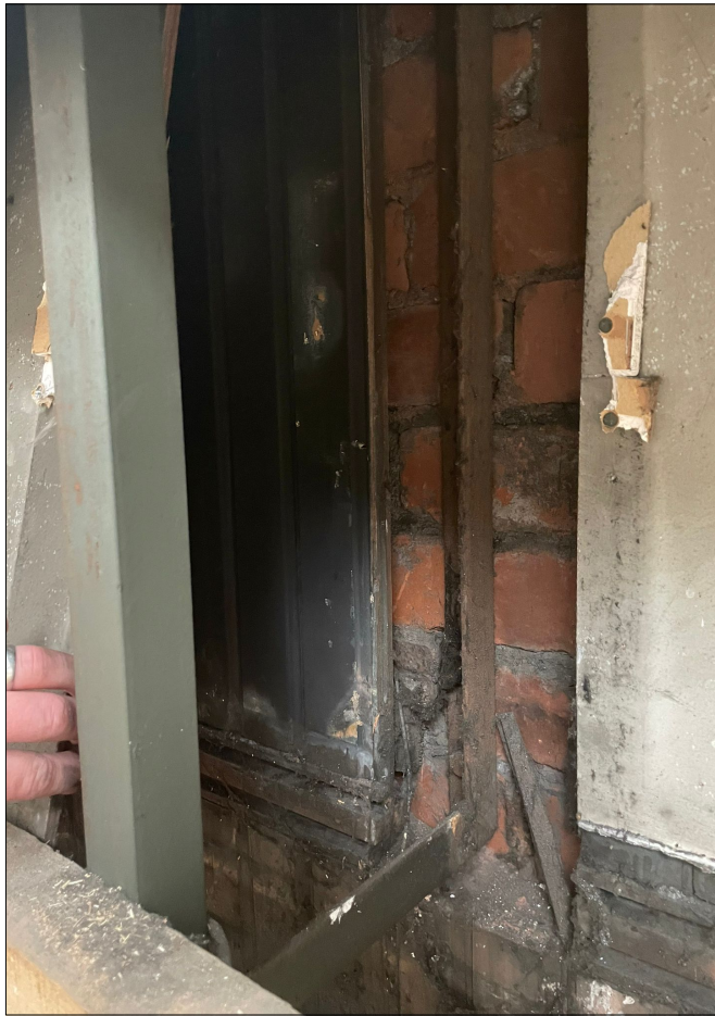
Image 03/04 - Close up image of existing cut through wall coverings for historic metal frame fixing points throughout gallery spaces. Historic cutting of wall covering has meant T&G / boarding has become less secure and is in poor condition as visible in images.
