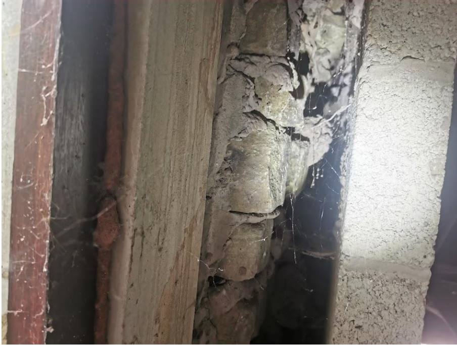
Photograph 11- Gap in wall of B2
