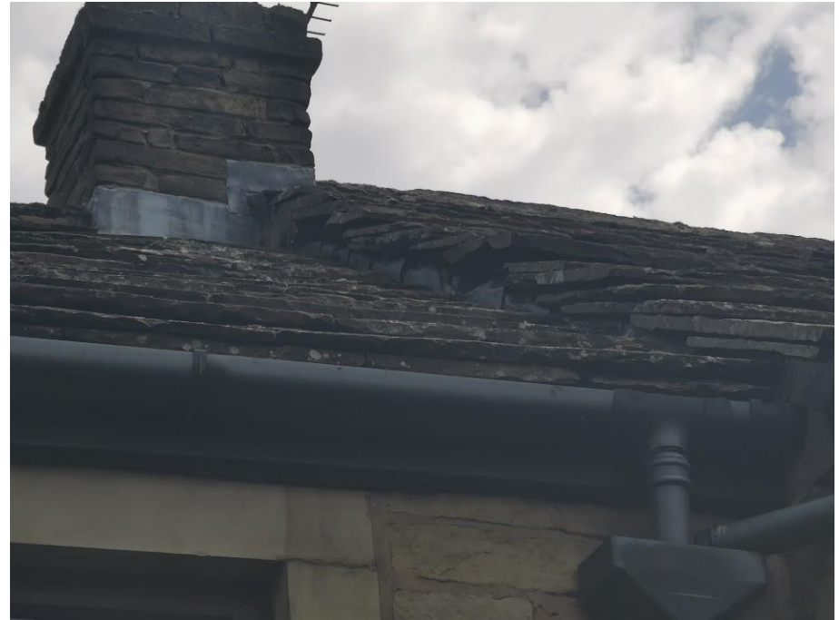
Photograph 2- Western elevation of B1, gaps under tiles and lining visible
