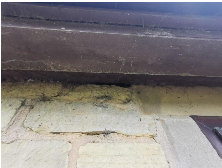
Photograph 7- Northern elevation, small gap in brickwork
