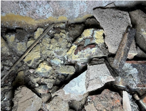
Fungal growth on building debris
