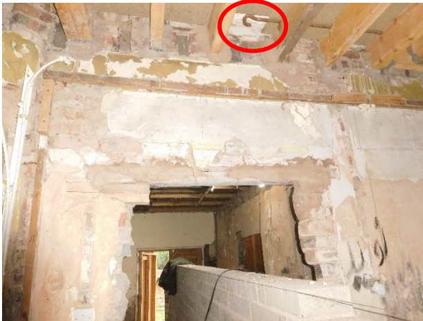
End of tie rod from lefthand elevation, righthand rod missing
