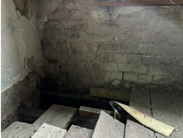
Cracking below landing window
