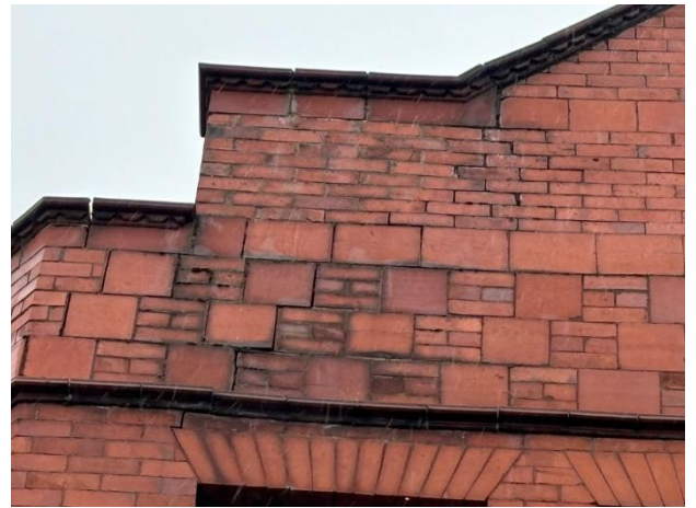
Cracking to parapet wall above second floor windows
