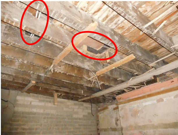
Holes in floor above
