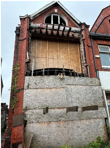
Missing front bay
