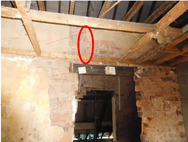
Cracking above doorway
