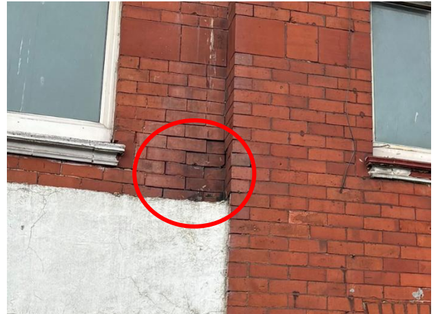
Distortion of brickwork above front door
