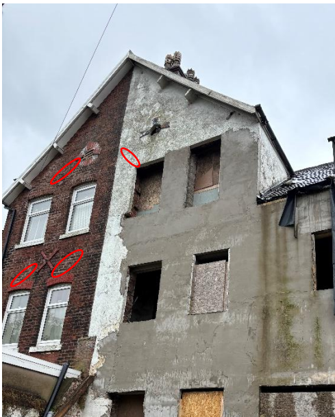
Cracking in rear wall of No.s 37 and 39
