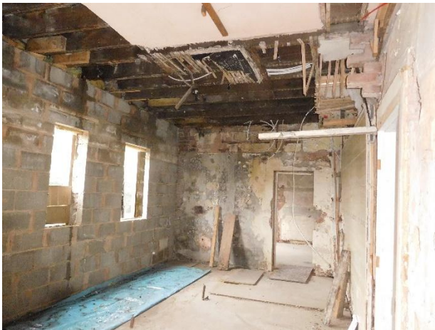
Water ingress along head of rear wall
