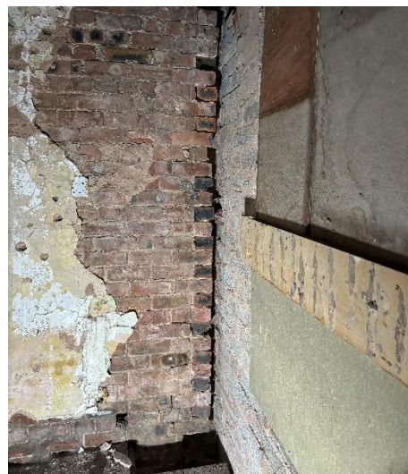
Lack of bonding between rear and internal walls
