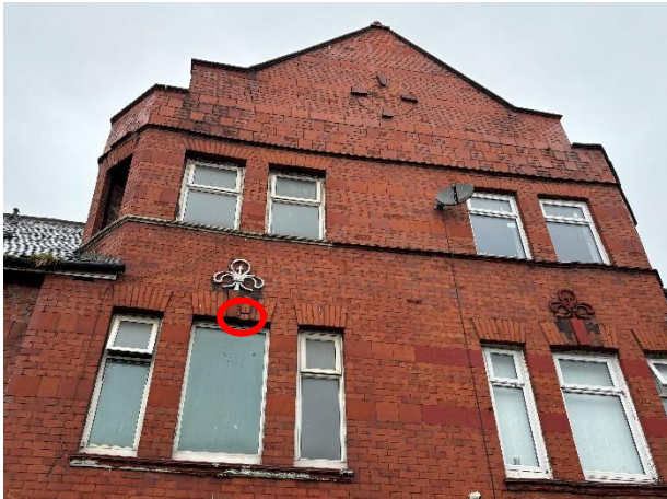
Dropped lintel over first floor window
