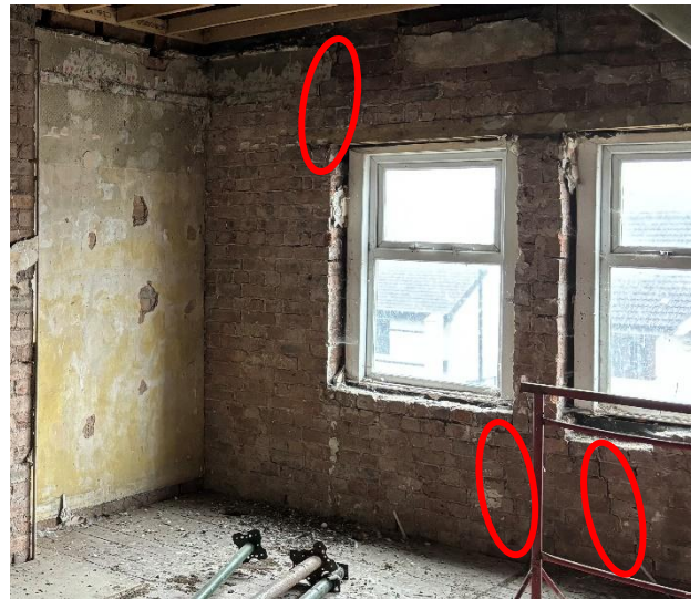
Cracking in front elevation
