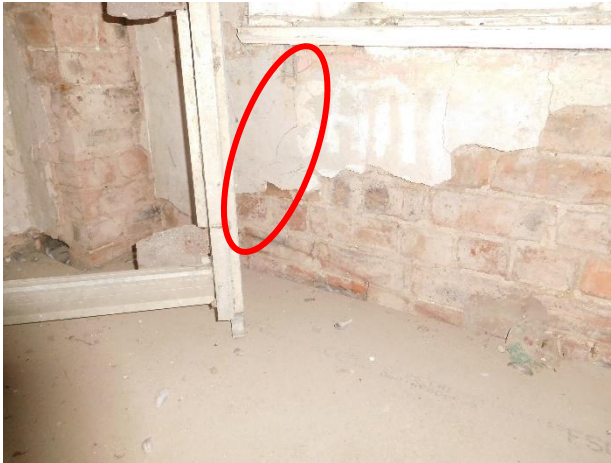
Cracking below front righthand room windows
