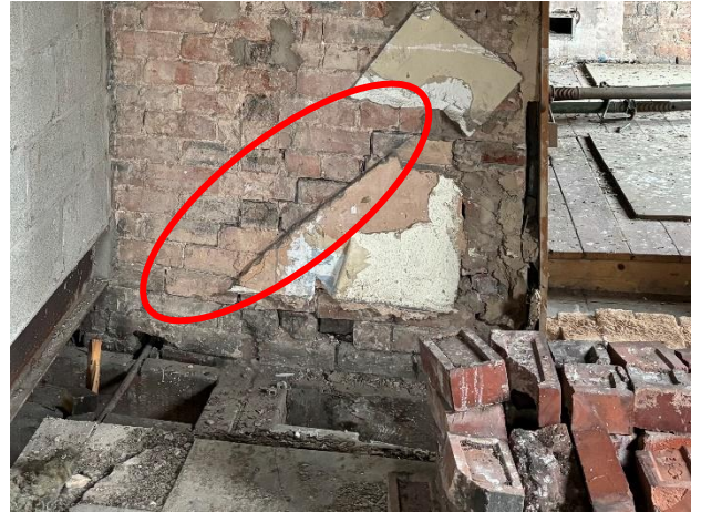
Cracking in wall between front rooms
