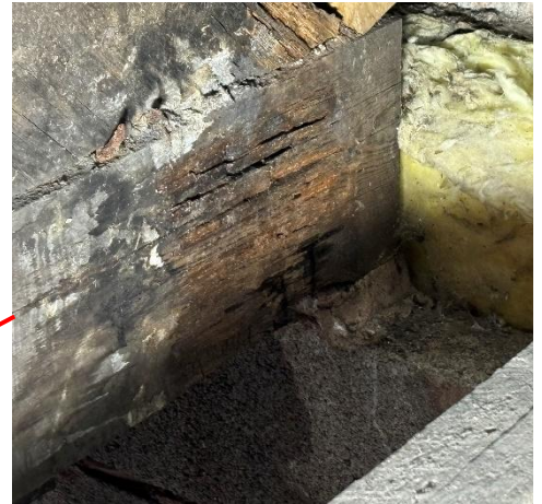
Wet rot in connection between principal rafter and beam
