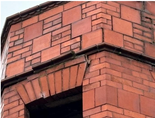
Rotated brick arch and cracking to parapet
