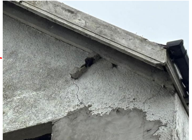
Rotten purlin end
