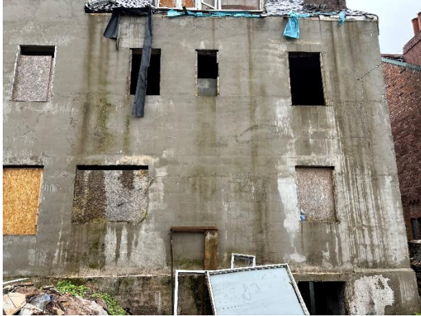
Water staining on rear wall
