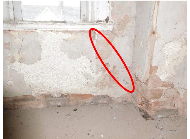
Cracking below front righthand room windows
