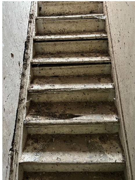
Stairs in very poor condition
