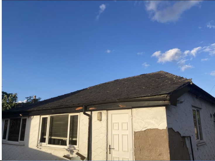
Photograph 5- Northern elevation showing the slate roof and damaged render, no features were evident on the rendered walls
