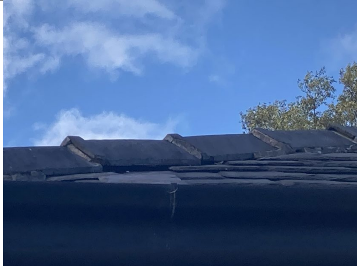
Photograph 6- northwest corner ridge line and hip showing missing mortar and small gaps between ridge tiles and slates, these features were rated as moderate and could not be fully inspected from the ground. They were all covered by the emergence surveys and NVA cameras.
