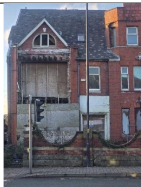
Front bay missing
