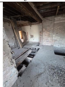
Holes in floor
