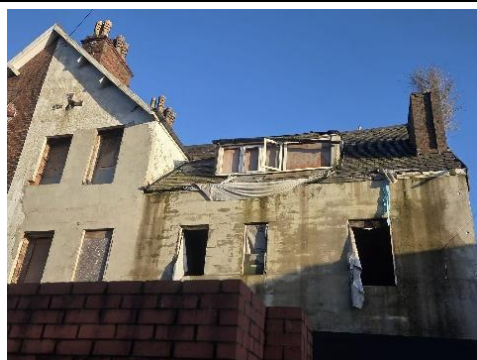
Evidence of water staining to the rear wall
