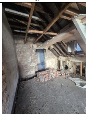
Masonry stored at second floor
