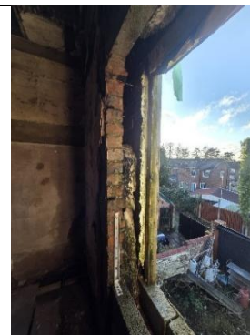
Internal evidence of water ingress to rear wall
