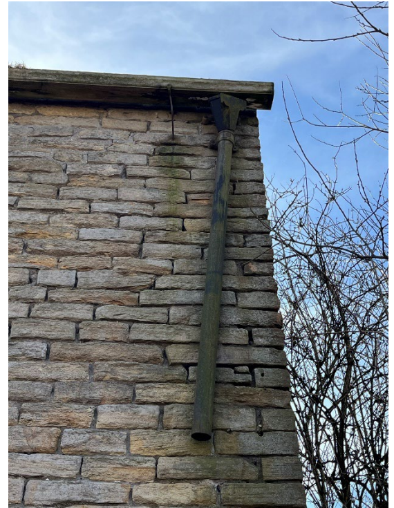
Figure 13 – Broken and rusting existing downpipe on the corner of the farmhouse
