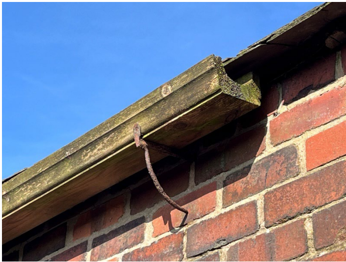
Figure 14 – Broken and rotting existing gutter on the former outbuildings supported by rusting brackets
