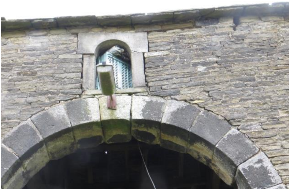
OPEN JOINTS TO SMALL WINDOW OVER ARCHED OPENING
