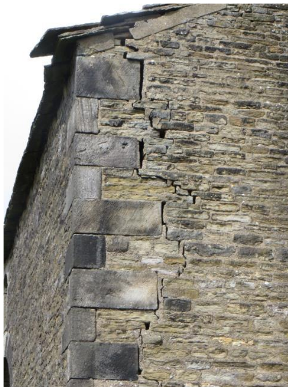
CRACK ADJACENT TO QUOINS TO FRONT CORNER
