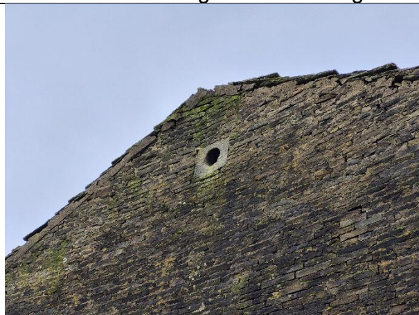
Photo 4: Hole in the wall of west facing side of building 1.
