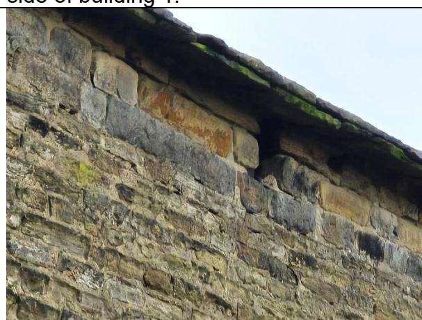
Photo 10: Hole in the northern facing wall of building 1.
