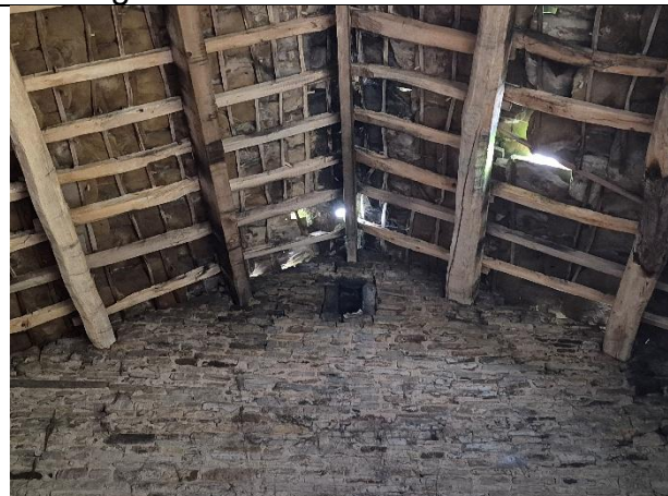
Photo 17: Holes in the roof of building 1.
