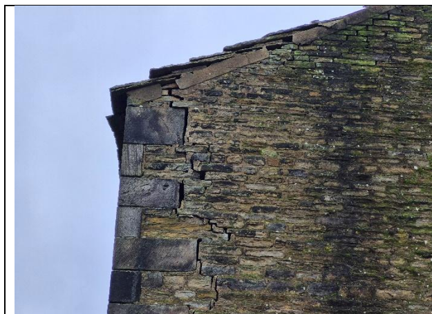
Photo 7: Missing mortar and gaps in tiles of east facing side.
