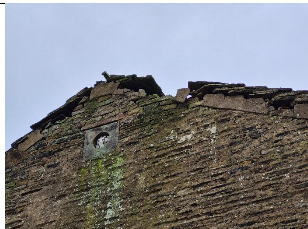
Photo 13: Missing tiles on eastern facing side of building 1.
