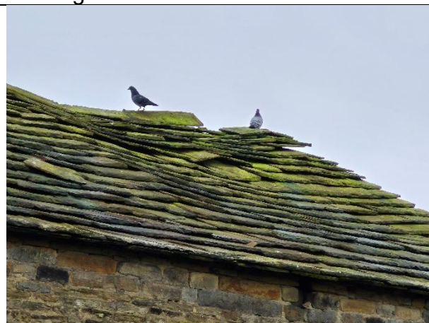
Photo 12: Gaps in tiles on northern facing roof.
