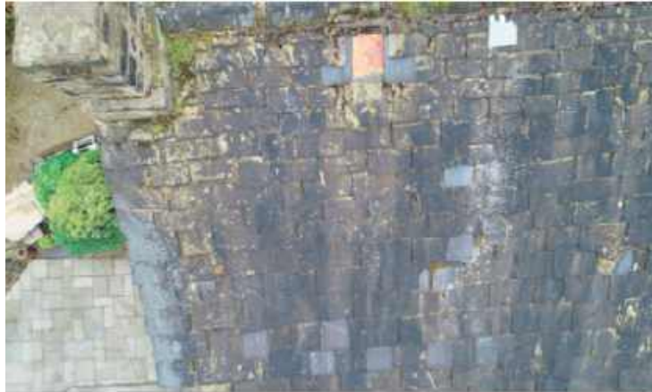
Photograph 8- Photograph from a previous roof structure survey showing the deteriorating roof structure
