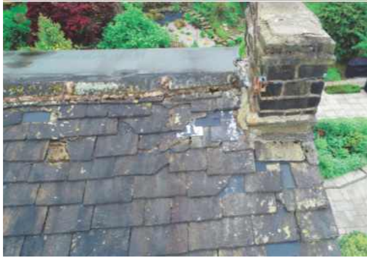
Photograph 7- Photograph from a previous roof structure survey showing the deteriorating roof structure
