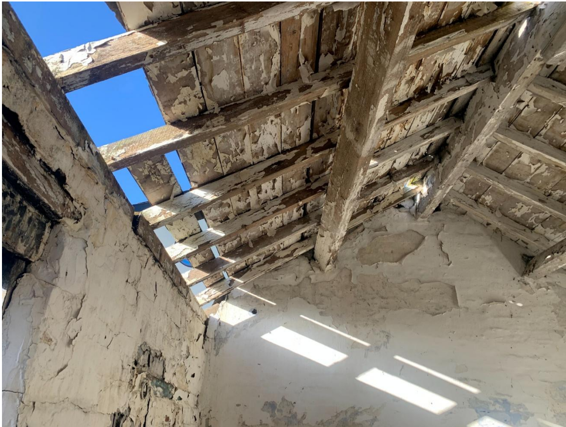
Plate 19: Gaps in roof.
