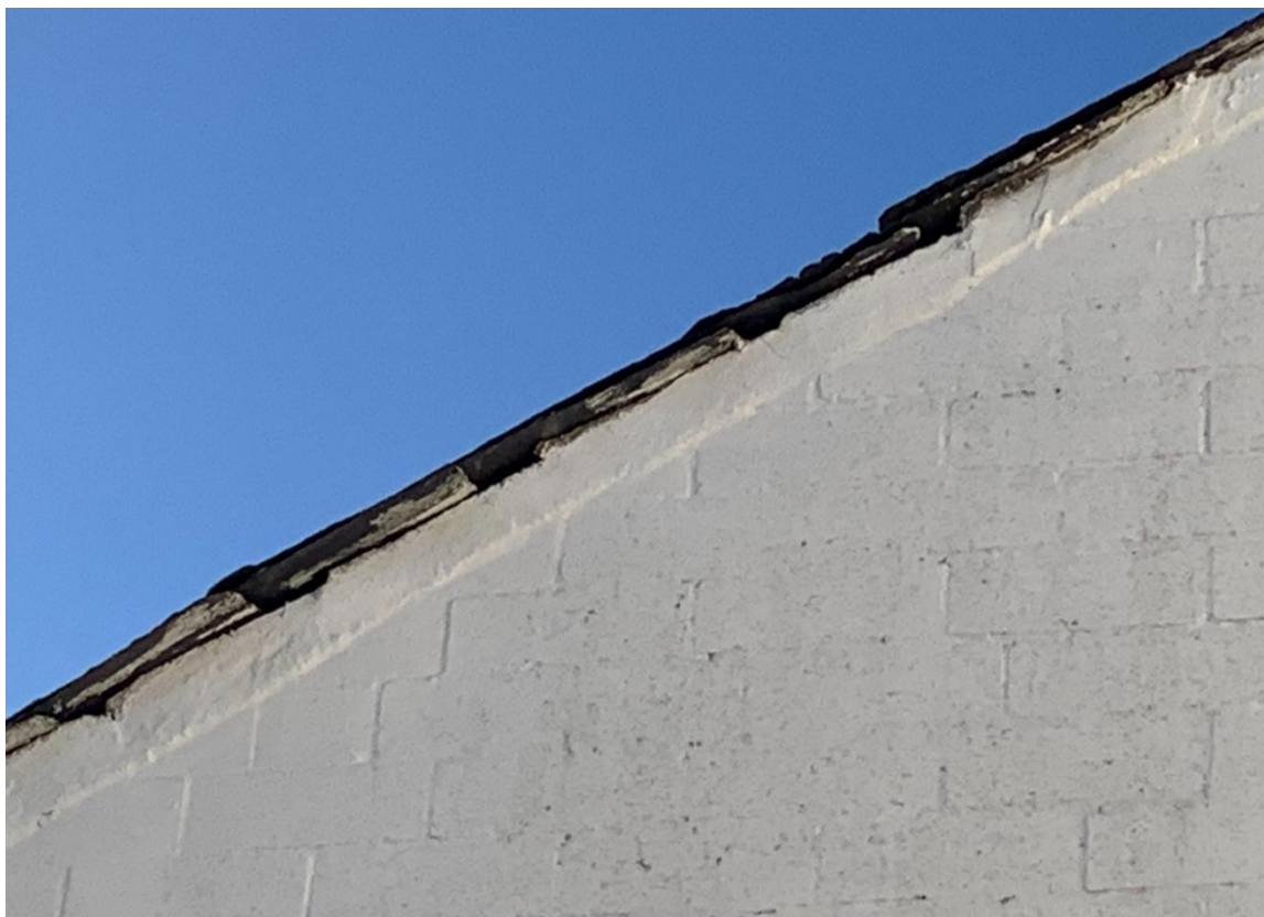
Plate 24: Gaps at roof edge.
