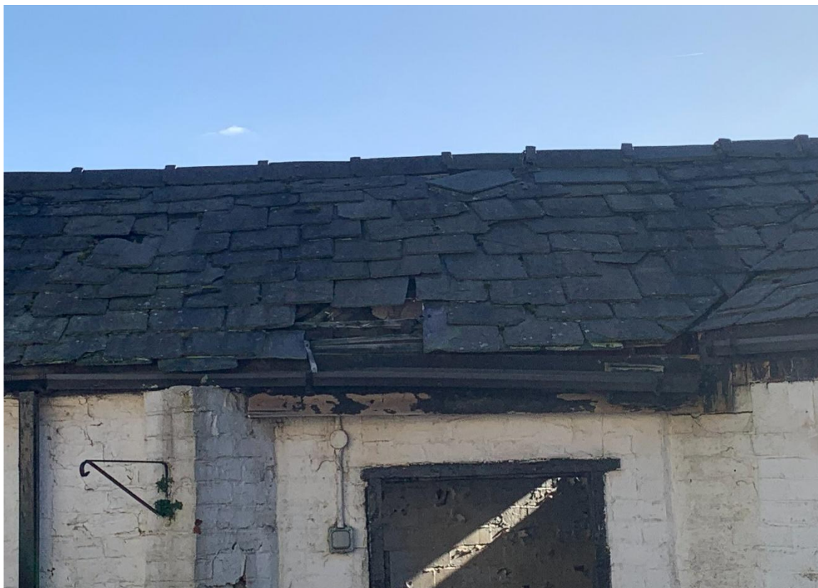
Plate 15: View of gaps in roof tiles.
