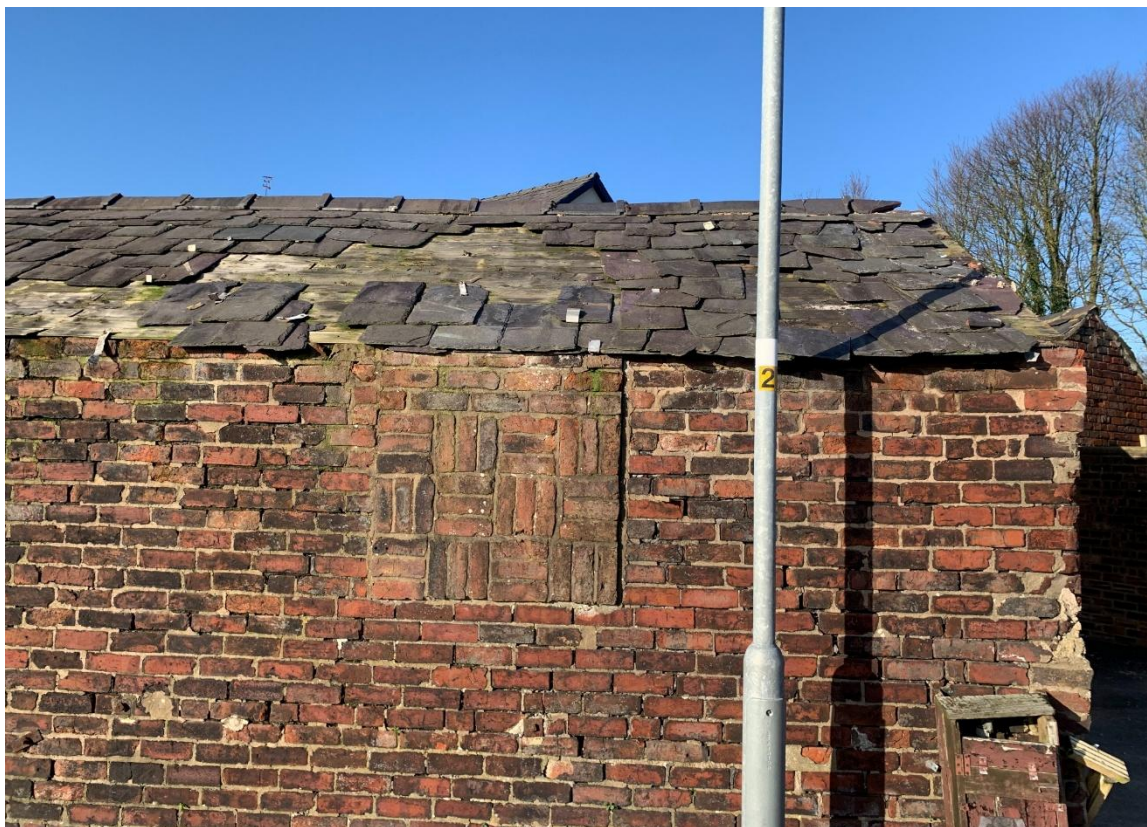
Plate 27: Dislodged and missing roof tiles.
