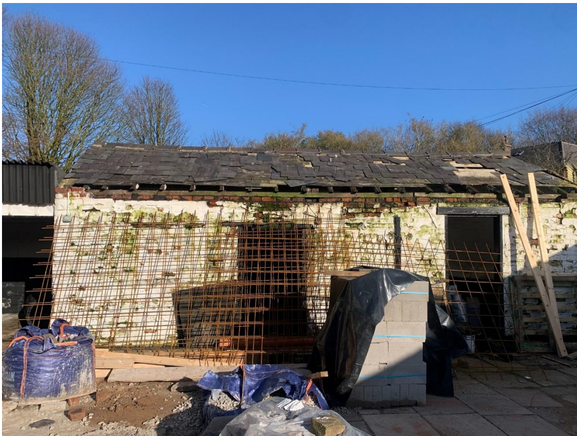
Plate 10: Several dislodged roof tiles are apparent.
