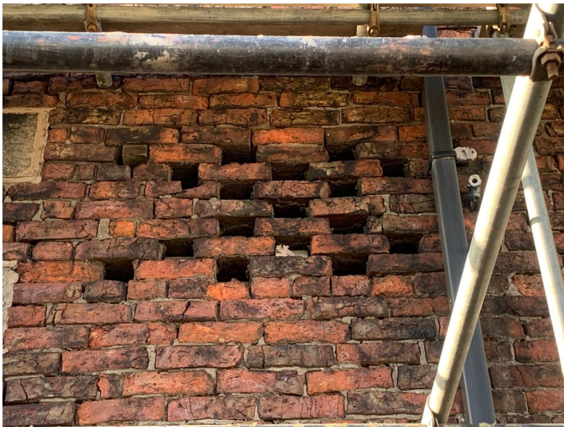
Plate 21: Gaps in brickwork.
