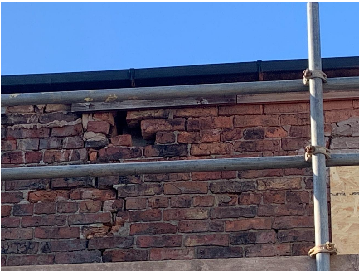
Plate 30: View of gaps in brickwork.
