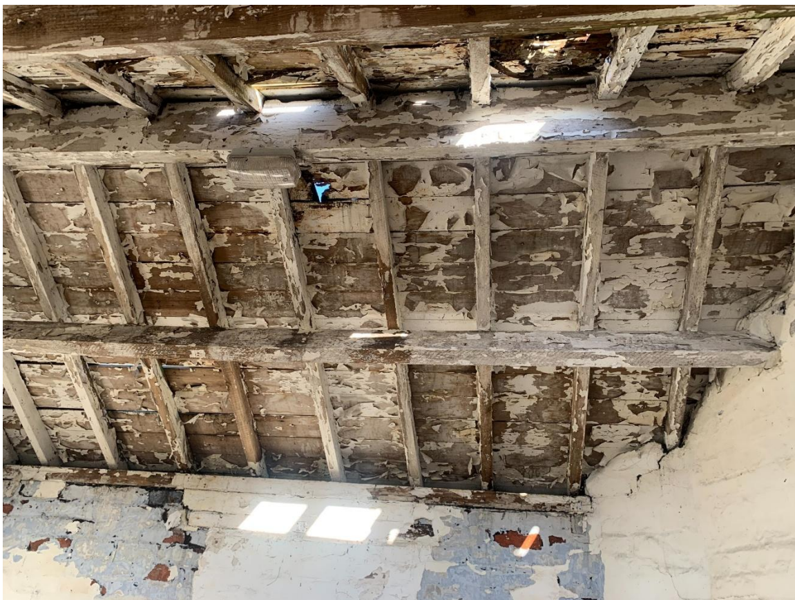
Plate 18: Gaps in roof.
