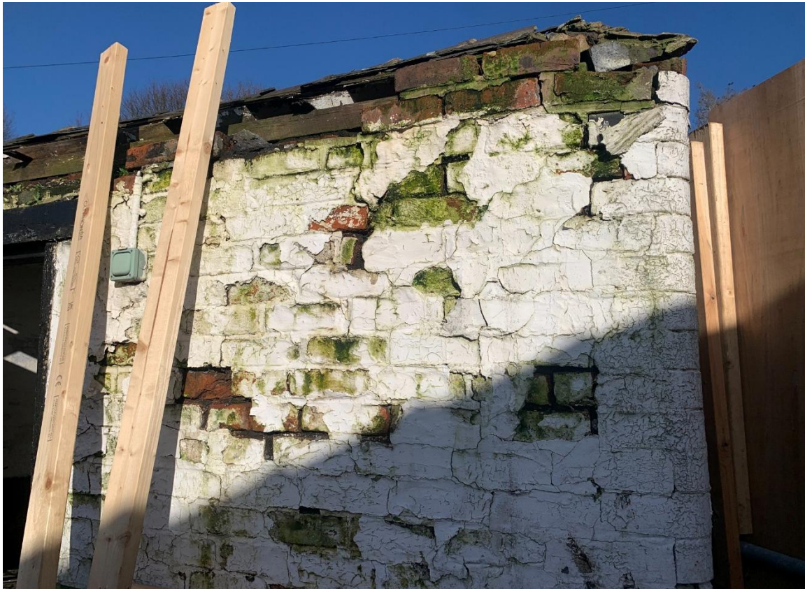
Plate 17: View of gaps suitable for bat access.
