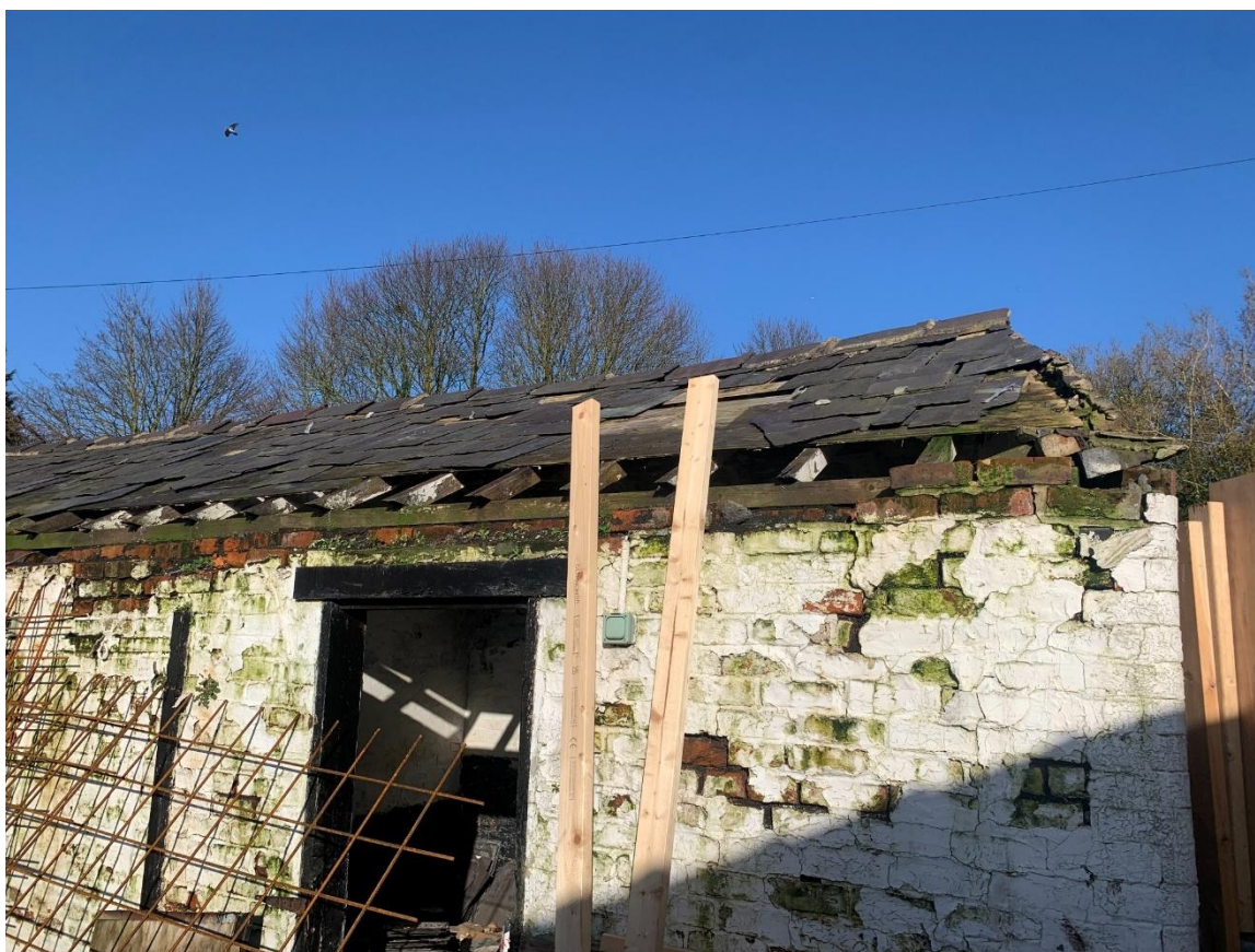
Plate 16: View of gaps in roof tiles and missing door (B3).
