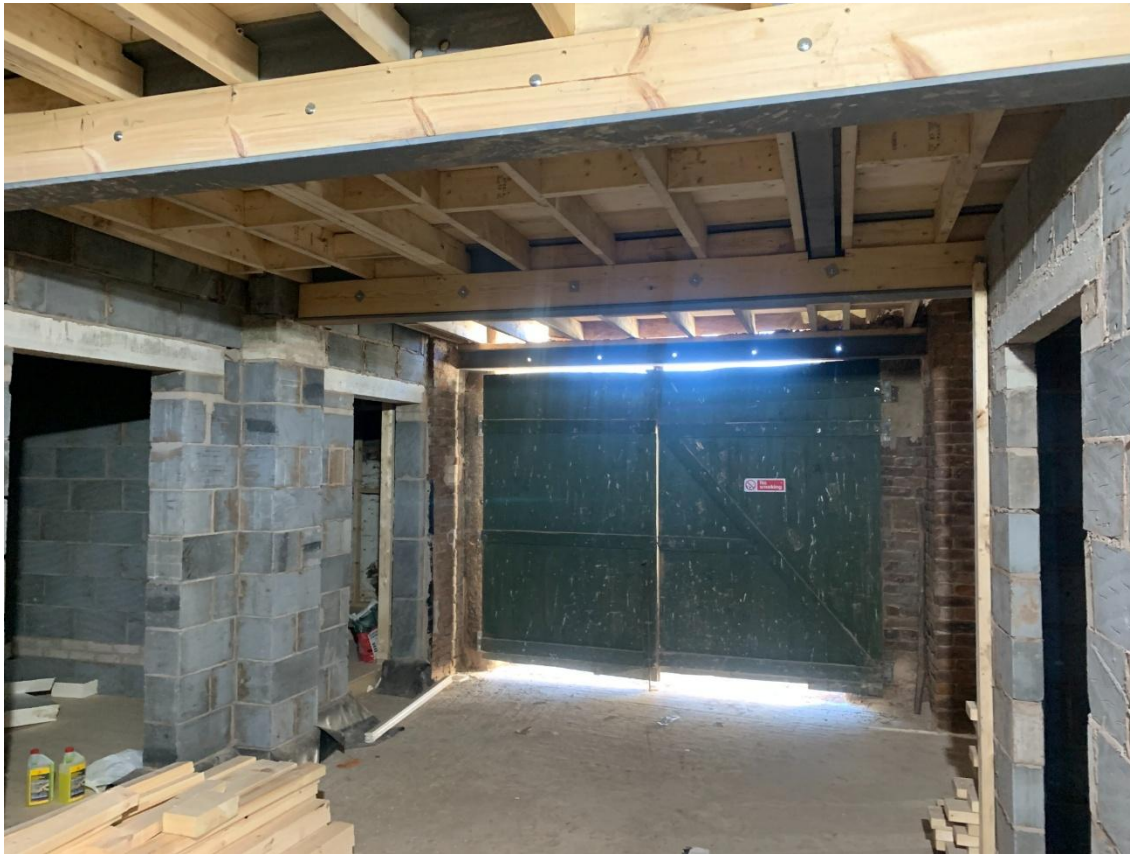
Plate 11: Gaps around door.
