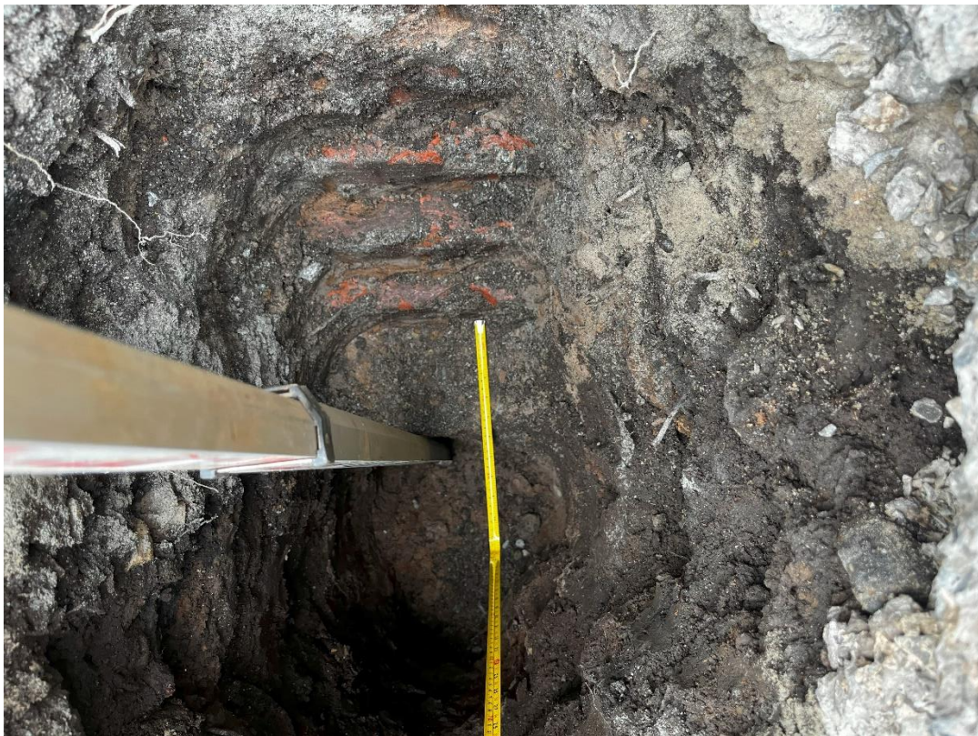
Plate 2 - HP01 concrete slab projects 270mm from the brick wall.
