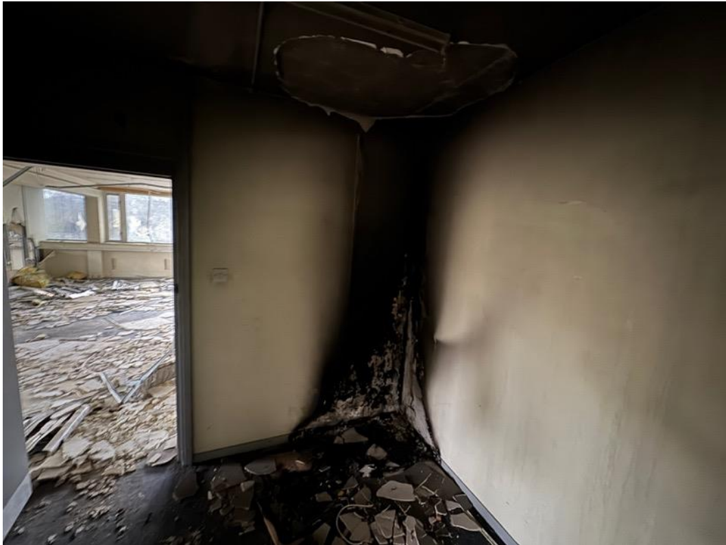
Image 88 – Fire damaged to central storeroom, looking toward the north.
