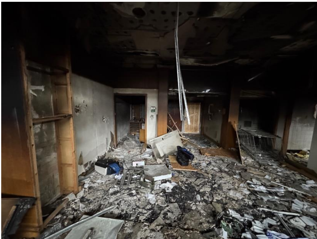
Image 41 – Internal view of main entrance lobby, small office space to left through archway. Extensive damage from arson and vandalism.
