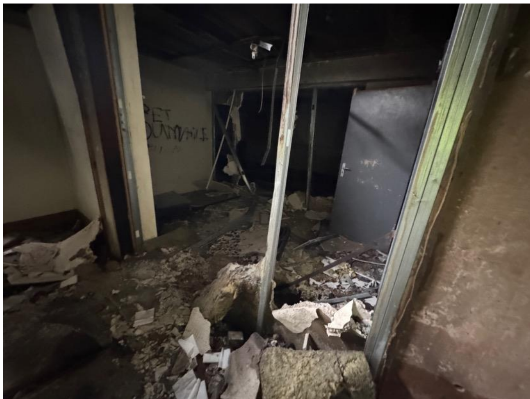
Image 45 – Internal view through ruined partition walls in extension to west side.
