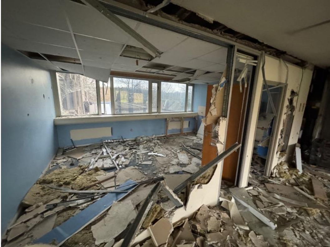
Image 68 – View into separate office, first floor, walls largely destroyed.
