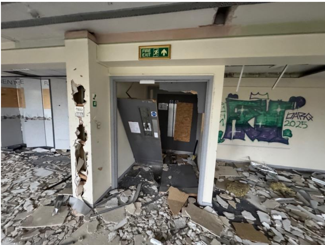
Image 93 – View of southern stairwell, second floor. Doors sealed shut preventing access.
