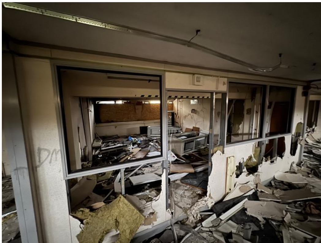
Image 55 – Office space to ground floor. Internal glazing missing and walls destroyed.
