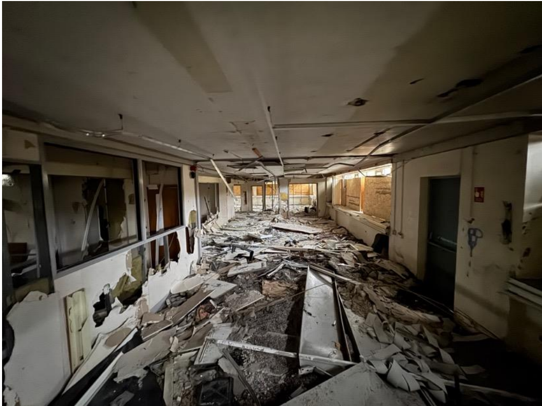
Image 58 – View to length of northern side of the ground floor, heavy piles of debris made access difficult.
