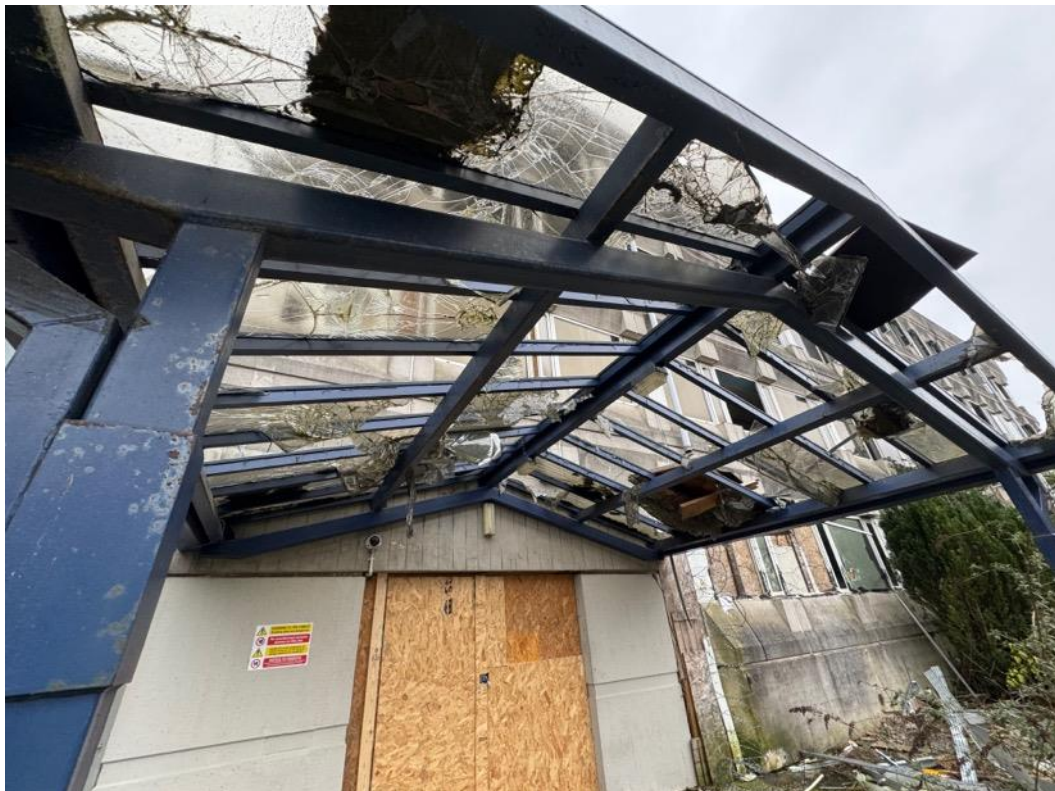
Image 39 – Closer view of glass canopy to main entrance, heavily vandalised. Original concrete block canopy lost at some stage.
