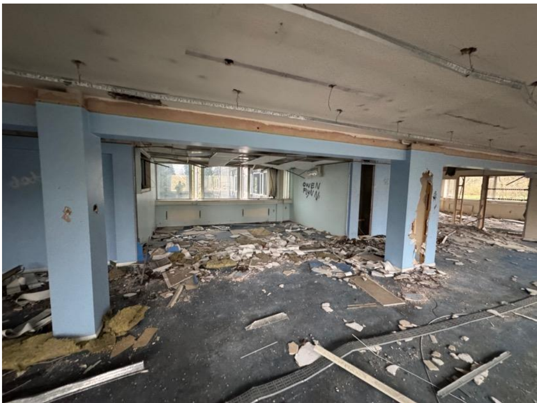
Image 73 – Former separate room to western edge first floor, partition wall now lost.
