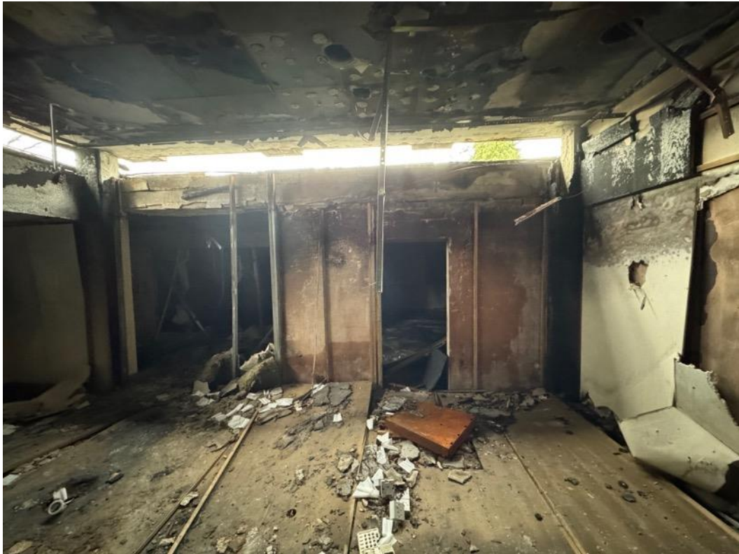
Image 44 – View of west wall of entrance hall. Wall finish largely collapsed onto floor, but some concrete panels visible.
