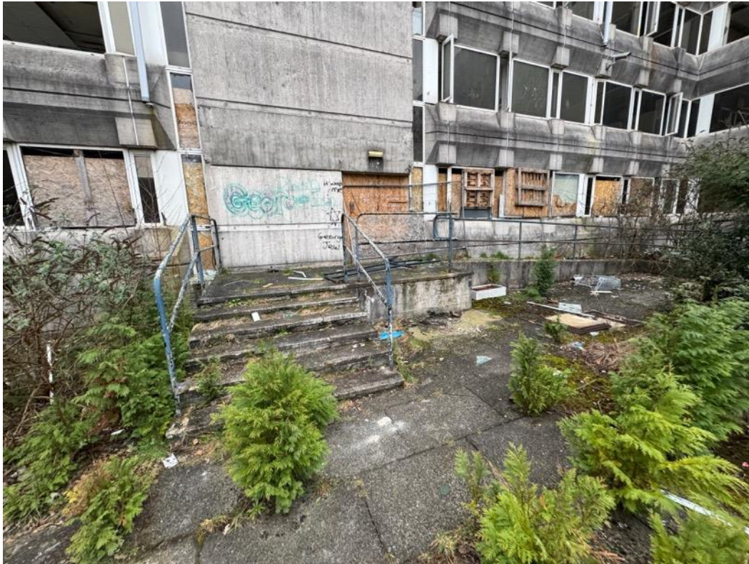
Image 26 – Closer view of access stairs and ramp to south elevation, doors have been boarded but once provided access to stairwell. Original concrete block canopy removed and not replaced.
