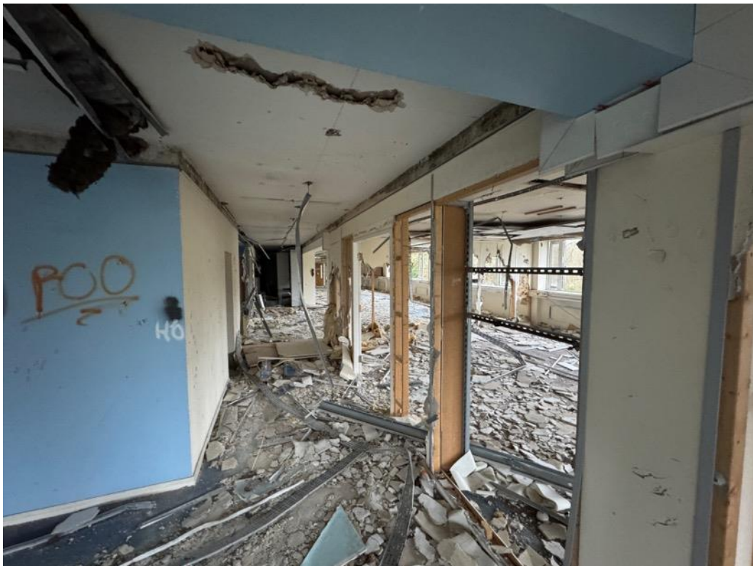
Image 71 – View to central corridor space, first floor. All partitions heavily damaged.
