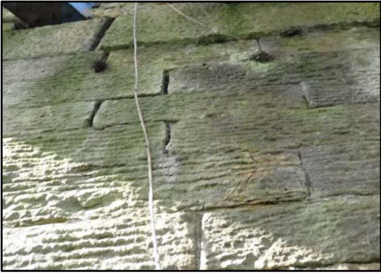
PHOTO SHOWING DEFECT 03 (01/09/2022)
