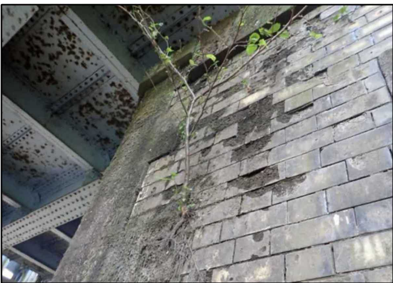
PHOTO SHOWING DEFECT 20 (01/09/2022)
