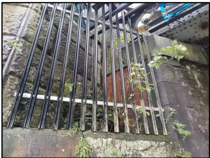
PHOTO 5 - STONE CORBEL BEHIND PALISADE FENCE
