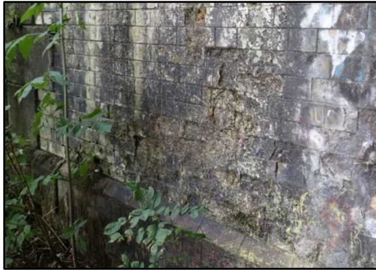
PHOTO SHOWING DEFECT 15 (01/09/2022)
