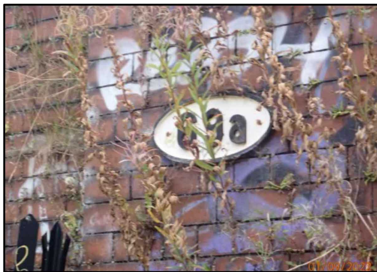
PHOTO SHOWING DEFECT 22&23 (01/09/2022)
