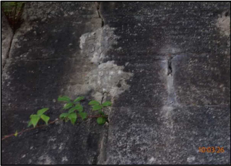
PHOTO SHOWING DEFECT 12 (01/09/2022)
