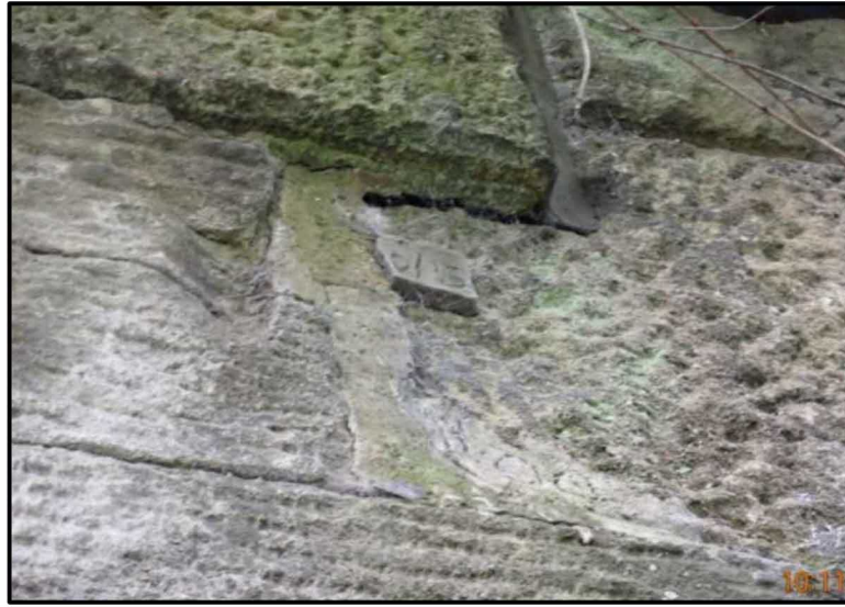
PHOTO SHOWING DEFECT 05 (01/09/2022)
