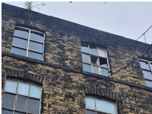
Photo 13: Broken window on B1 fourth storey.
