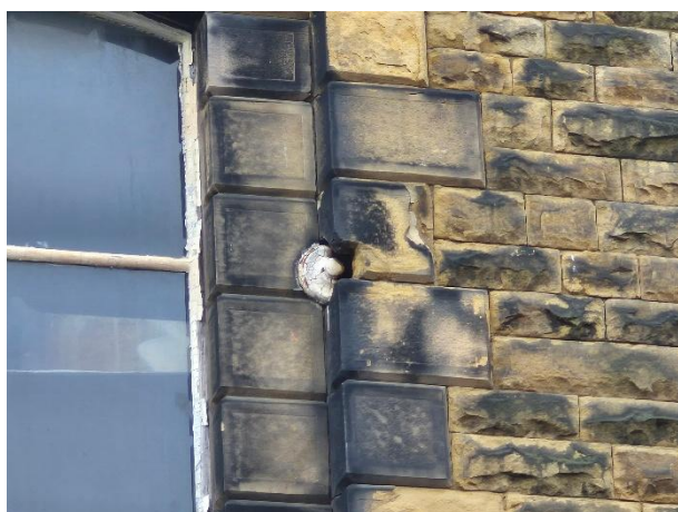
Photo 15: Hole in wall on B1 second storey.
