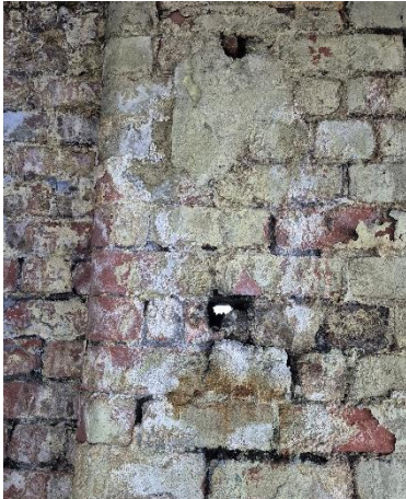
Photo 31: Interior wall of fourth story with holes and gaps in brickwork.
