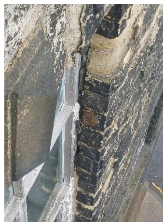
Photo 20: Missing mortar around windows on B1.
