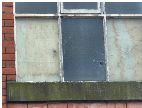
Photo 12: Broken window on B1 second storey.
