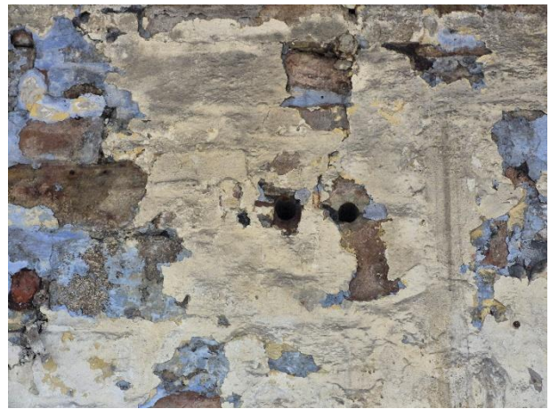
Photo 34: Interior wall of fourth story with holes and gaps in brickwork.
