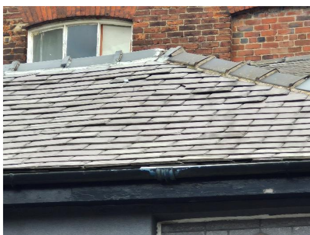
Photo 21: Lifted roof tiles on B2.
