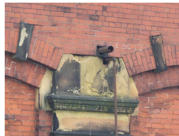
Photo 18: Gaps around pipe on B1.2.
