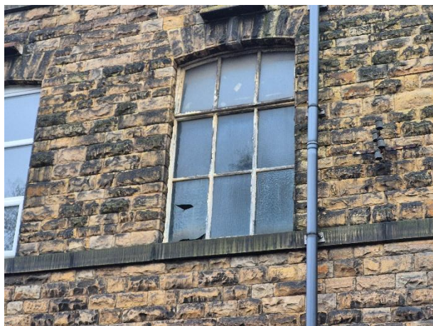
Photo 11: Broken window on B1 second storey.
