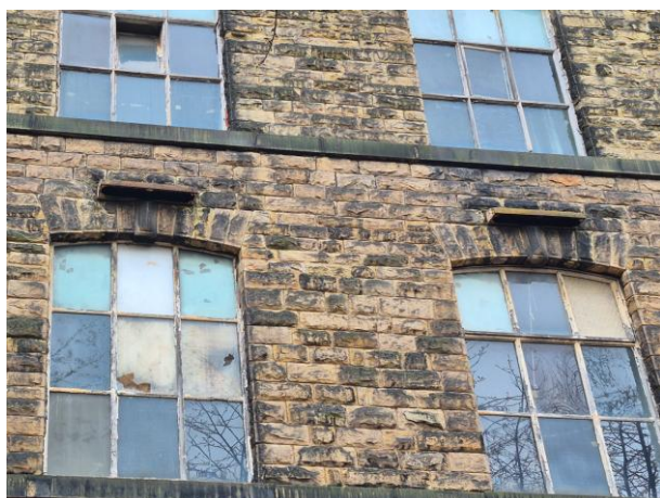
Photo 17: Vent openings above second storey windows. Jackdaws seen entering/exiting.
