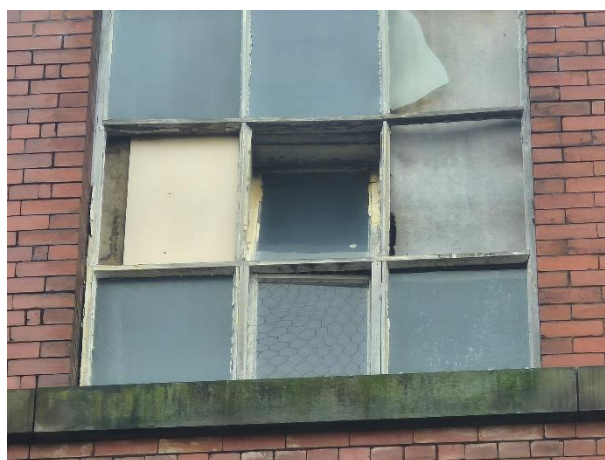
Photo 16: Gap in window boards on B1 fourth storey.
