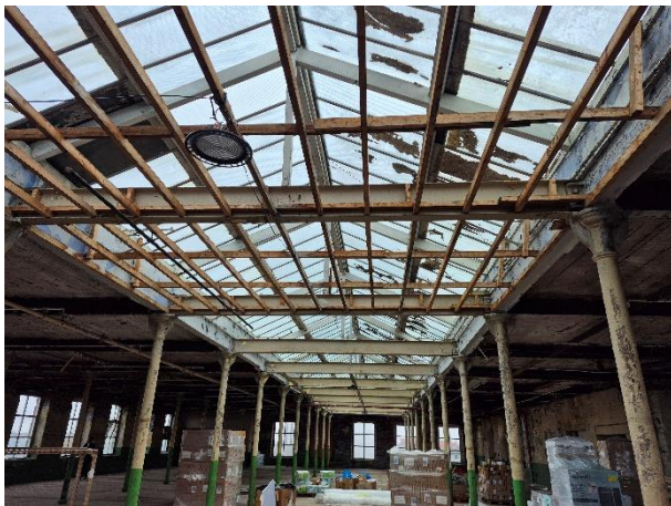
Photo 27: B1 fourth storey ceiling.
