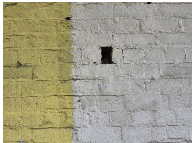
Photo 36: Interior wall of fourth story with holes and gaps in brickwork.
