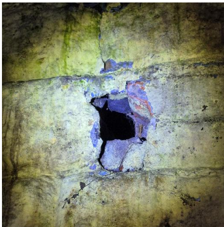
Photo 33: Interior wall of fourth story with holes and gaps in brickwork.
