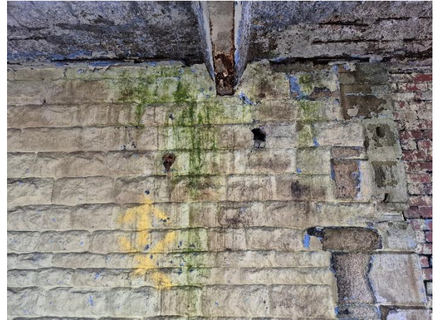
Photo 32: Interior wall of fourth story with holes and gaps in brickwork.
