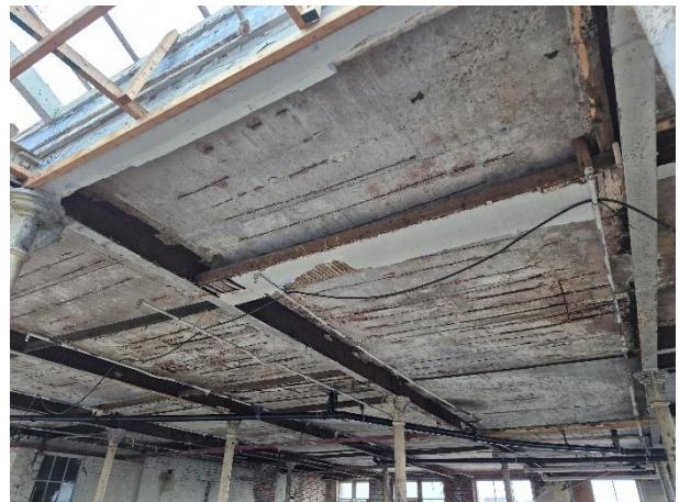
Photo 28: B1 fourth storey ceiling.
