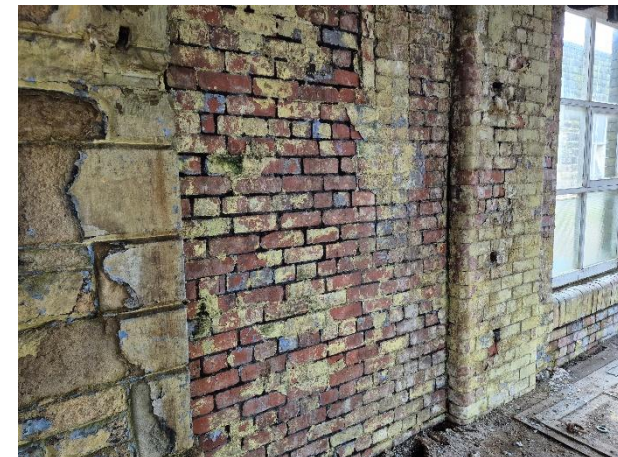
Photo 30: Interior wall of fourth story with holes and gaps in brickwork.
