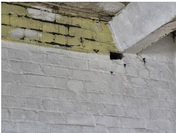
Photo 35: Interior wall of fourth story with holes and gaps in brickwork.
