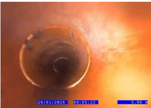
7, 00:00:39, 6.00 m Joint displaced, medium (between 1.0 and 1.5 times the pipe wall thickness)
