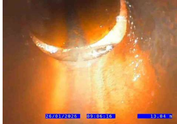
18, 00:01:32, 13.10 m Joint displaced, large (over 1.5 times the pipe wall thickness)
