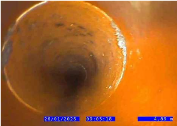
5, 00:00:35, 4.90 m Encrustation, light at joint from 12 o'clock to 12 o'clock
