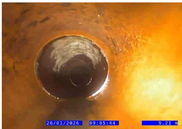
13, 00:01:00, 9.35 m Joint displaced, medium (between 1.0 and 1.5 times the pipe wall thickness)
