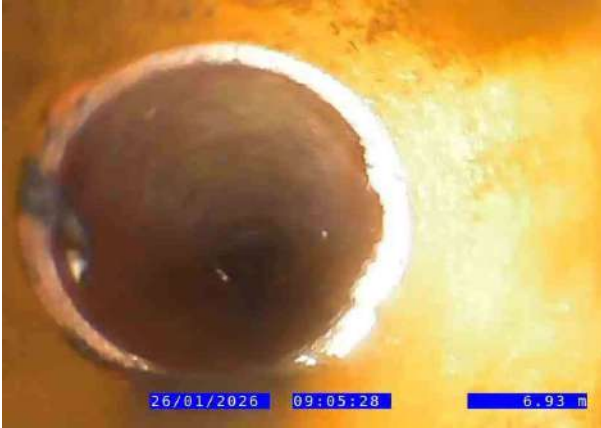
9, 00:00:44, 7.00 m Joint displaced, large (over 1.5 times the pipe wall tickness)
