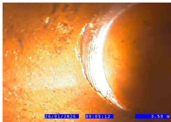
4, 00:00:28, 3.60 m Crack, circumferential at joint from 6 o'clock to 10 o'clock
