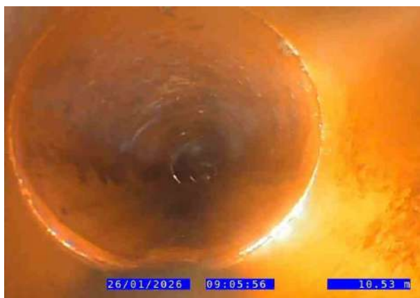
15, 00:01:12, 10.55 m Joint displaced, medium (between 1.0 and 1.5 times the pipe wall thickness)
