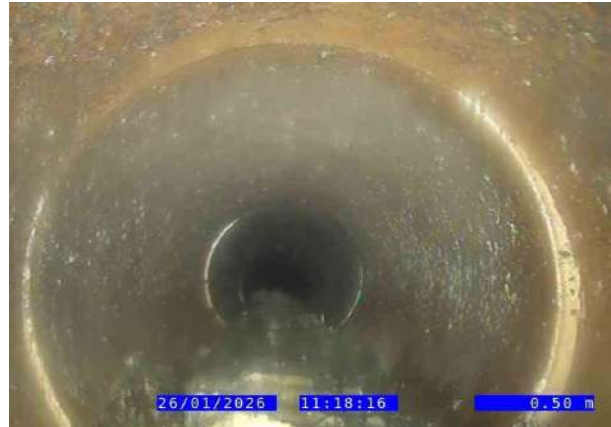
2, 00:00:00, 0.00 m Encrustation, heavy from 6 o'clock to 6 o'clock, start
