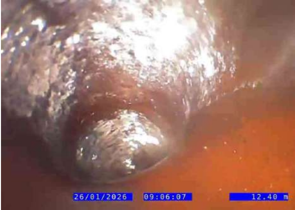
17, 00:01:24, 12.40 m Encrustation, medium from 12 o'clock to 12 o'clock, start
