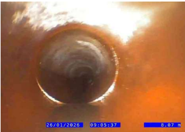
11, 00:00:53, 8.20 m Joint displaced, medium (between 1.0 and 1.5 times the pipe wall thickness)
