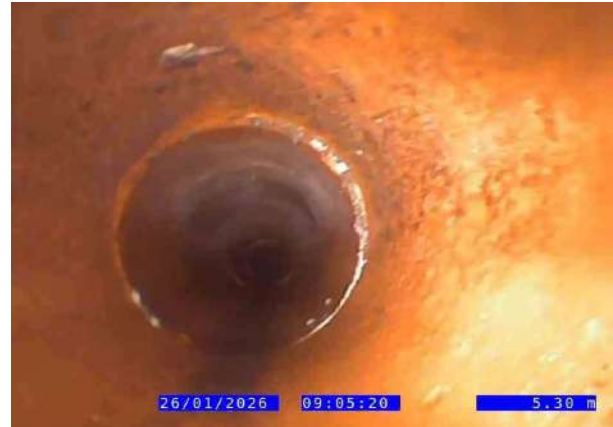
6, 00:00:37, 5.50 m Joint displaced, medium (between 1.0 and 1.5 times the pipe wall thickness)
