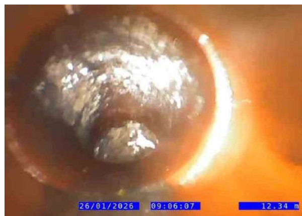
16, 00:01:23, 12.34 m Joint displaced, medium (between 1.0 and 1.5 times the pipe wall thickness)
