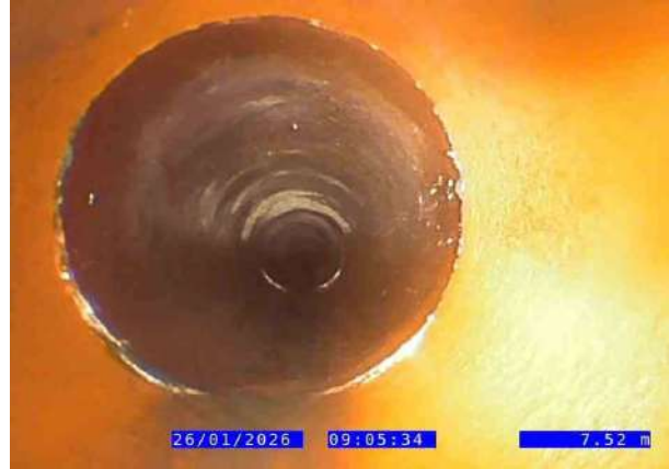
10, 00:00:51, 7.60 m Joint displaced, medium (between 1.0 and 1.5 times the pipe wall thickness)
