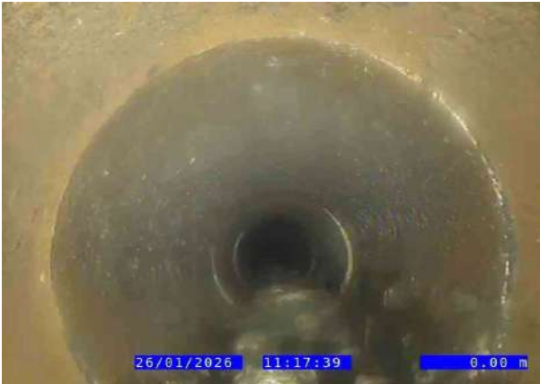
1, 00:00:00, 0.00 m Encrustation, heavy from 6 o'clock to 6 o'clock, start
