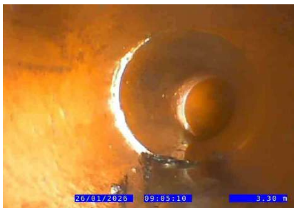
3, 00:00:26, 3.50 m Joint displaced, medium (between 1.0 and 1.5 times the pipe wall thickness)
