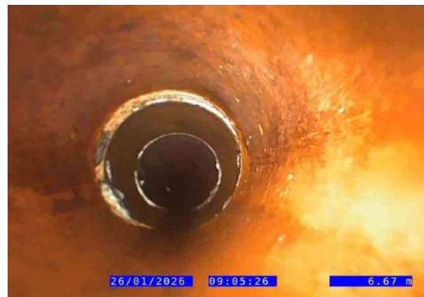
8, 00:00:43, 6.80 m Joint displaced, large (over 1.5 times the pipe wall thickness)
