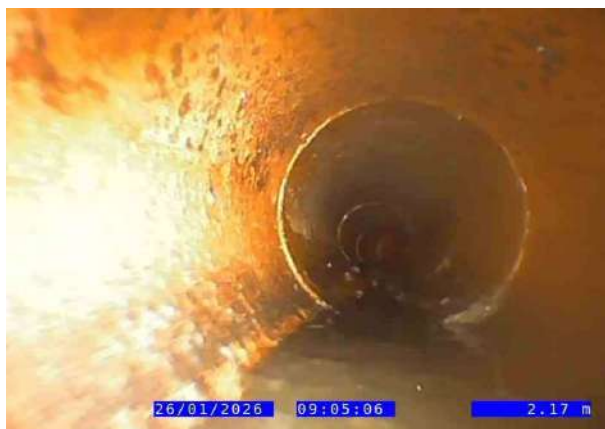
1, 00:00:22, 2.30 m Encrustation, medium at joint from 4 o'clock to 7 o'clock
