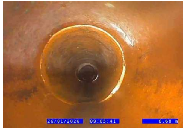
12, 00:00:58, 8.70 m Joint displaced, medium (between 1.0 and 1.5 times the pipe wall thickness)
