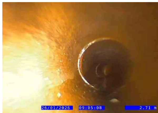
2, 00:00:24, 2.80 m Joint displaced, medium (between 1.0 and 1.5 times the pipe wall thickness)
