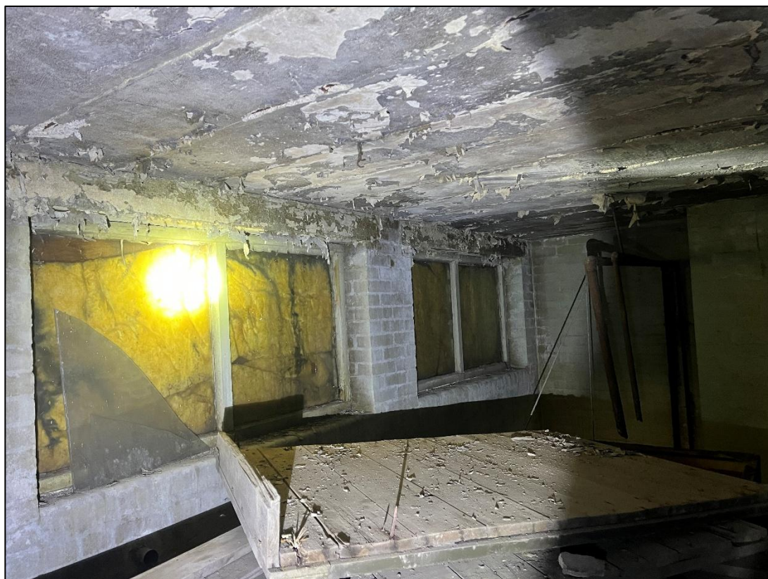
Plate 7 – Further view of plant room
