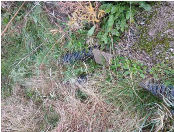
Photo 7 — Drainage running through the ditch.
